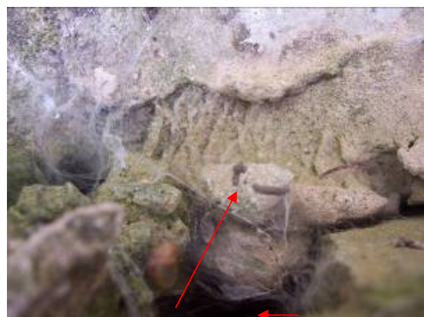
Location of bat droppings outside crevice on southern parapet wall
