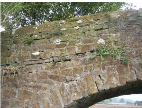
Upper parapet wall showing cracks and crevices
