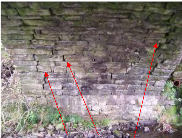
Underneath the bridge looking west showing the numerous cracks where mortar is failing
