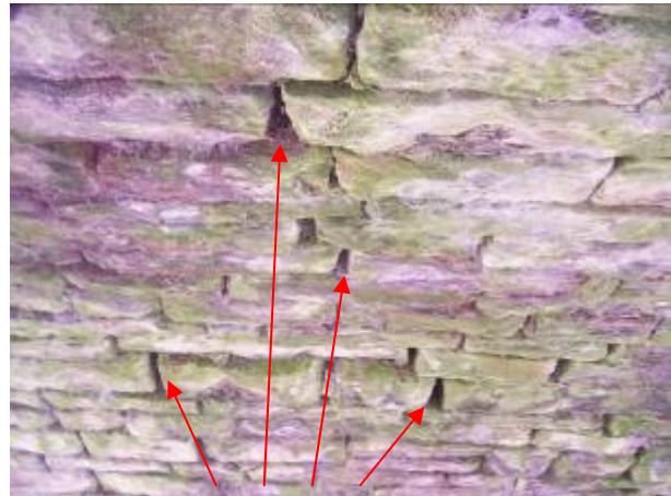
Underneath the bridge span showing some of the numerous cracks where mortar is failing
