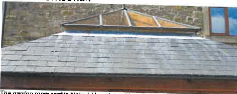
The garden room roof is hipped blue slate with a glazed top section. The eaves overhang having timber fascias and soffits.
