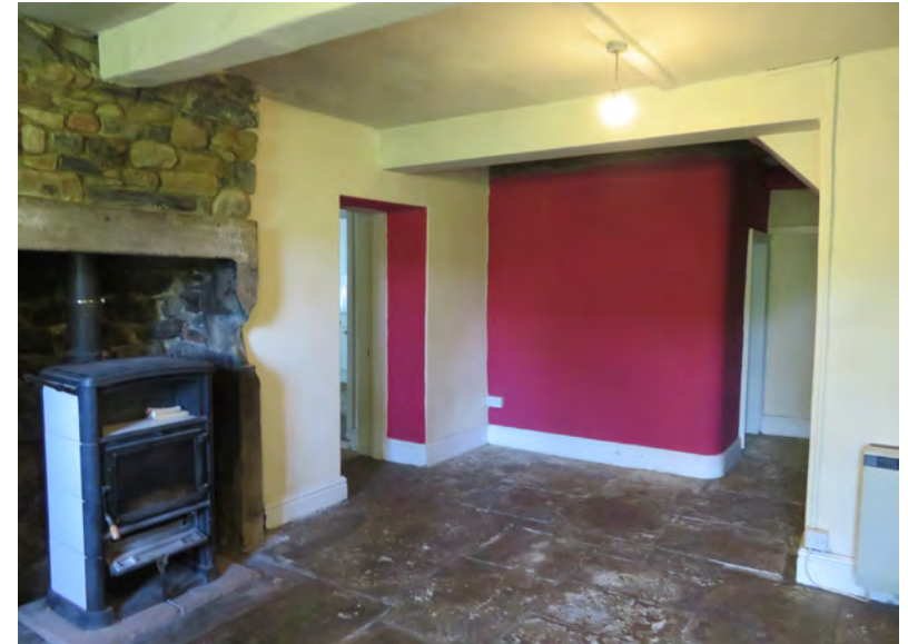
Cottage Living Room showing the pantry wall at the rear which is proposed to be removed.
