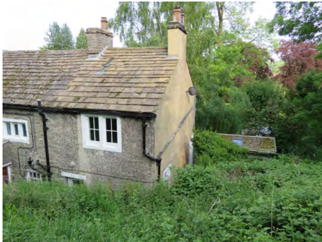
View to the SW gable of the cottage showing the roof of the Garden Room and the external toilet is concealed structure within the retaining wall.
