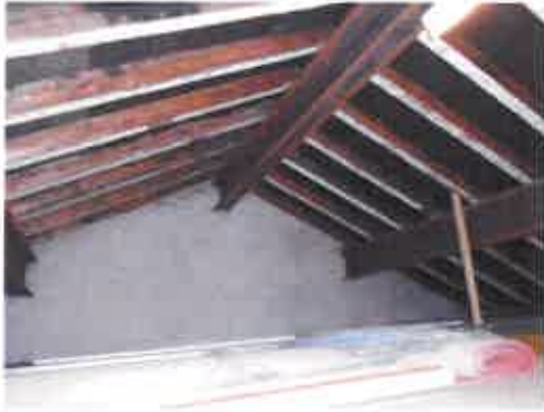
Garage roof void was steel purlins, timber rafters, and felt underlay. The ceiling joists were boarded.
