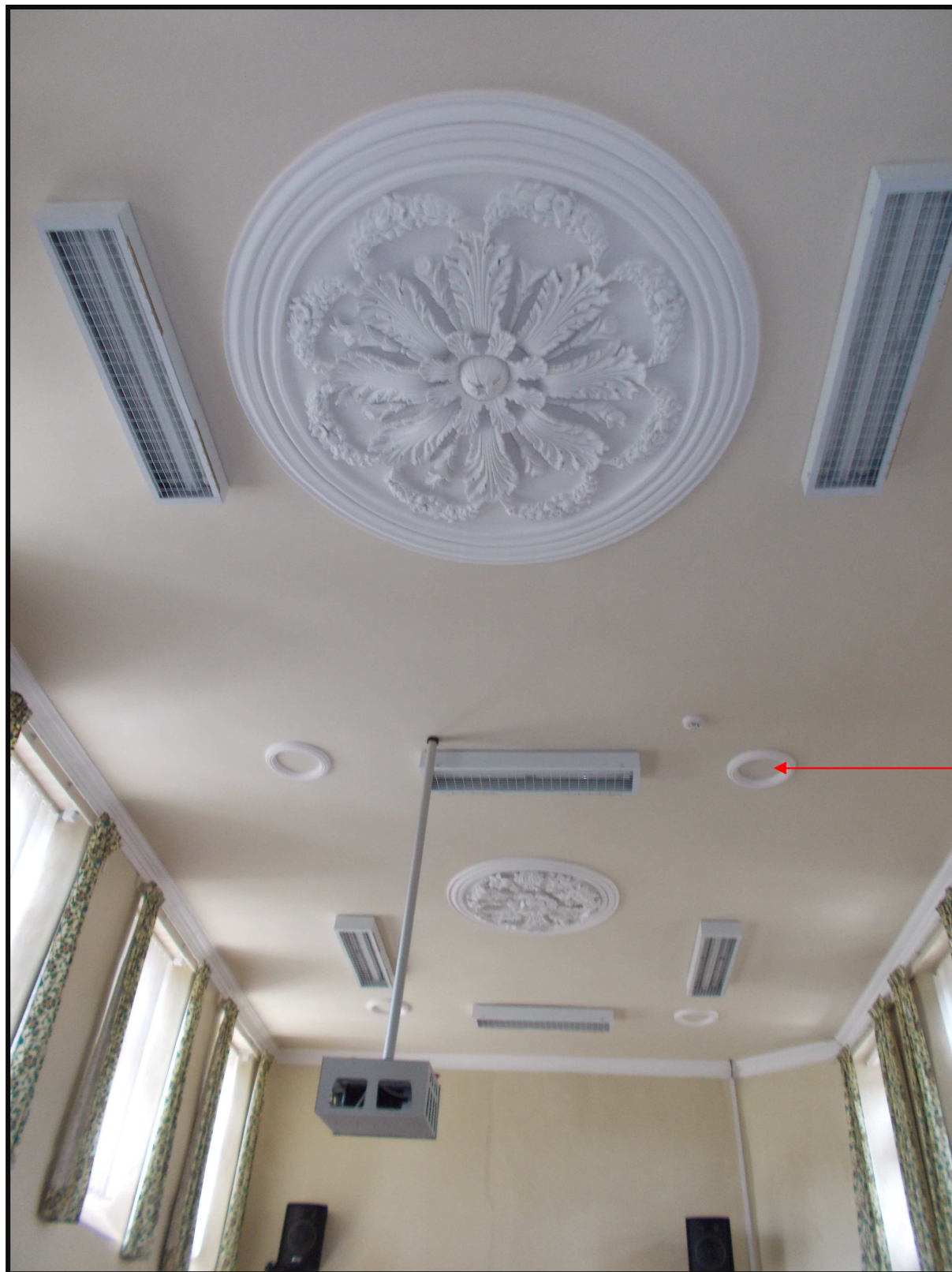
Figure 4 - Represents the existing plaster moulding detail where diffusers are to be installed
