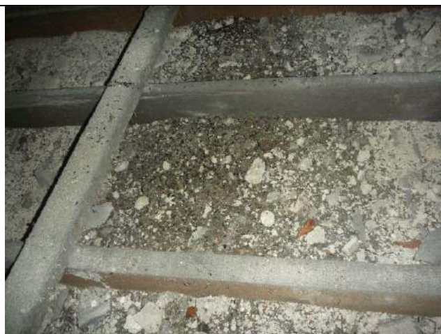
Photo 31: Roost 7, 1000's droppings under the ridgeline, with clusters of droppings located at the south-east facing gable
