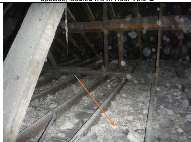
Photo 36: Roost 10 as indicated by the orange arrow, 30+ old droppings, indicative of pipistrelle bats, located within Roof Void I4.
