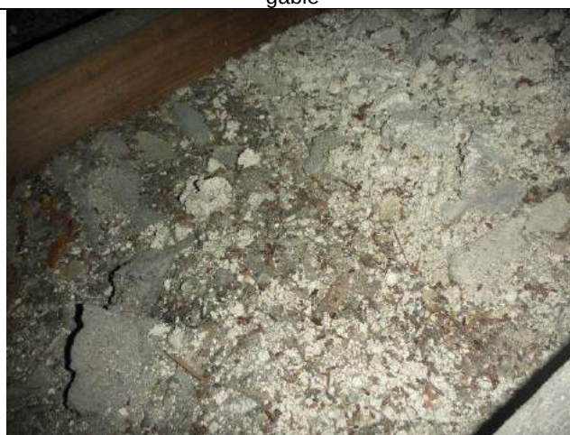
Photo 33: Roost 8, 1000's droppings under the ridgeline, with clusters of droppings located at the south-east facing gable
