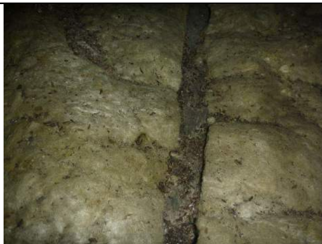
Photo 29: Roost 5, 50+ droppings along length of ridge beam of Roof Void B4
