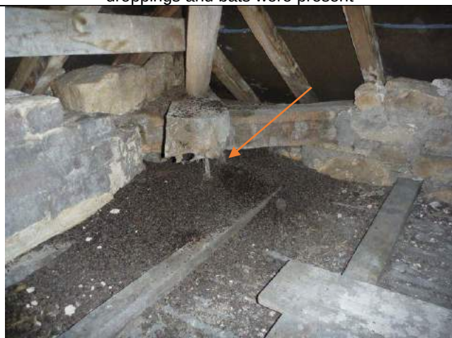
Photo 26: Roost 2, 1000's droppings present at north-western corner of Roof Void B1
