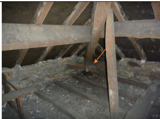
Photo 24: Roost 1 location, as indicated by orange arrow. Roost located at south-eastern of Roof Void B1. 1000's of droppings and bats were present
