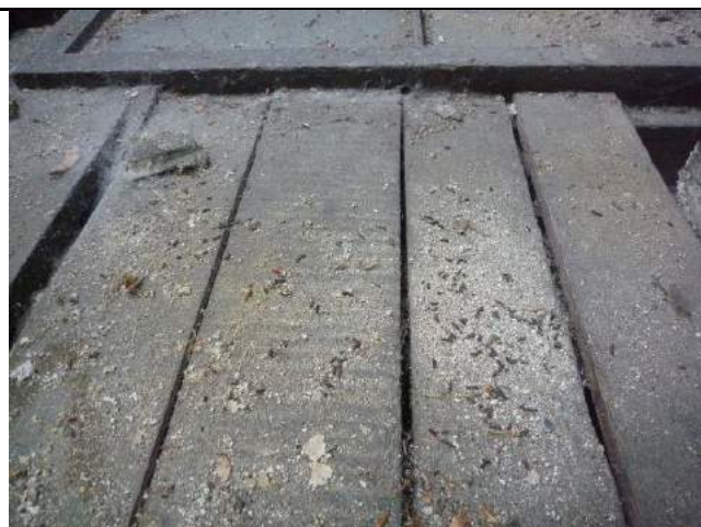
Photo 34: Roost 9, 30+ droppings indicative of a pipistrelle species, located within Roof Void I2
