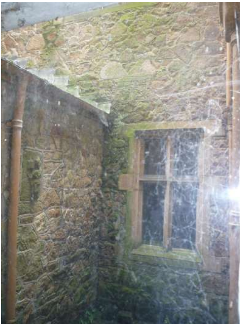
10. Mullion window of 1875 from inner yard, 1892 cross passage infill on left. Note Roman relief carving of goddess (To be relocated).
