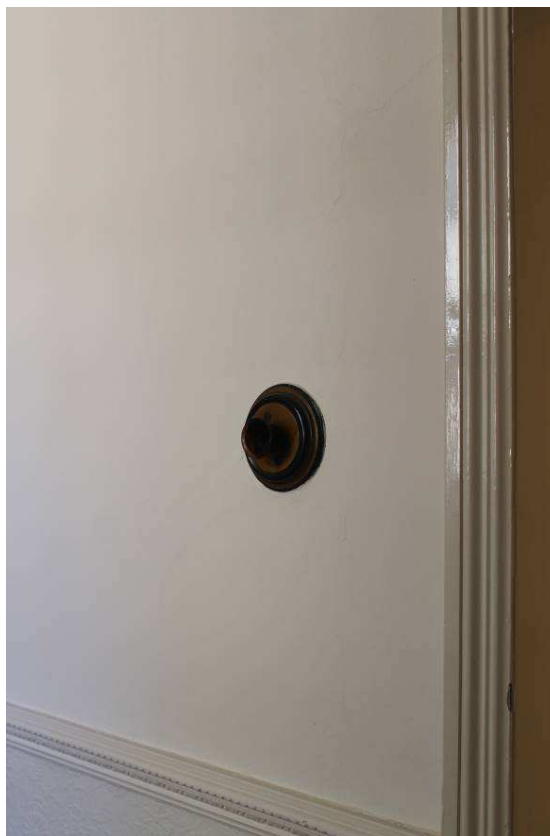
Plate 24: Intercom system, on west wall of corridor Room F14a
