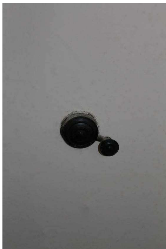
Plate 44: Service bell in corridor Room F18
