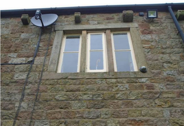
Figure 5: Window Replacements - Ref: W1 - W3. Two fixed casement windows to either side, of a central window with side hung opening casement.
