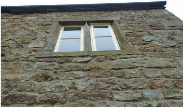
Figure 7: Window Replacements - Ref: W6 - W7. Left hand side - fixed casement window. Right hand side window with side hung opening casement.
