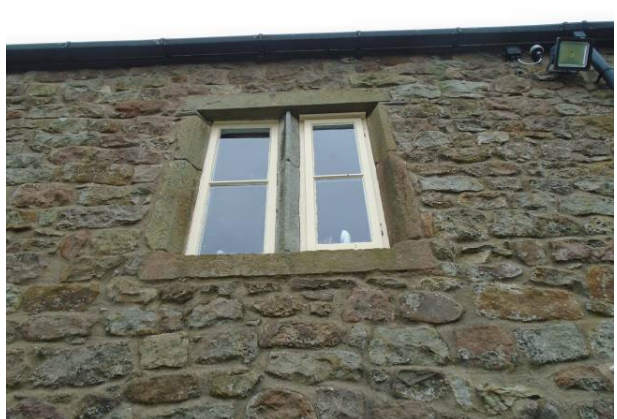
Figure 6: Window Replacements - Ref: W4 - W5. Left hand side - fixed casement window. Right hand side window with side hung opening casement.
