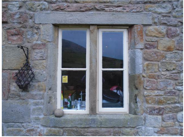
Figure 8: Window Replacement - Ref: W8 & W9. Left hand side - fixed casement window. Right hand side window with side hung opening casement.
