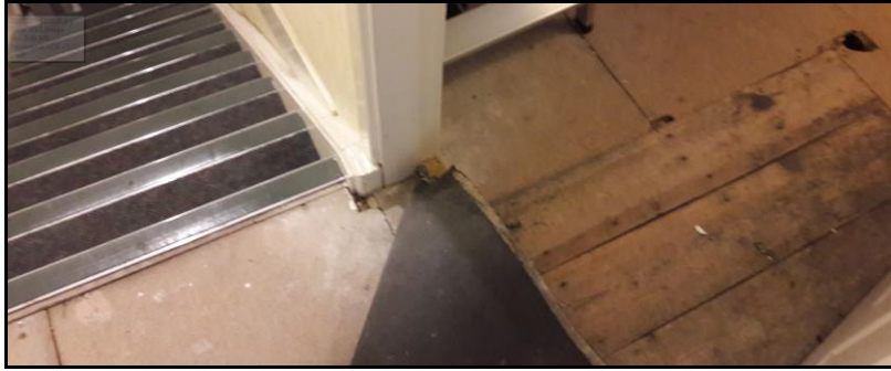
Figure 1. Alterations to the floor at the head of the stair (first floor level) with new chipboard panel and plank boarding.
