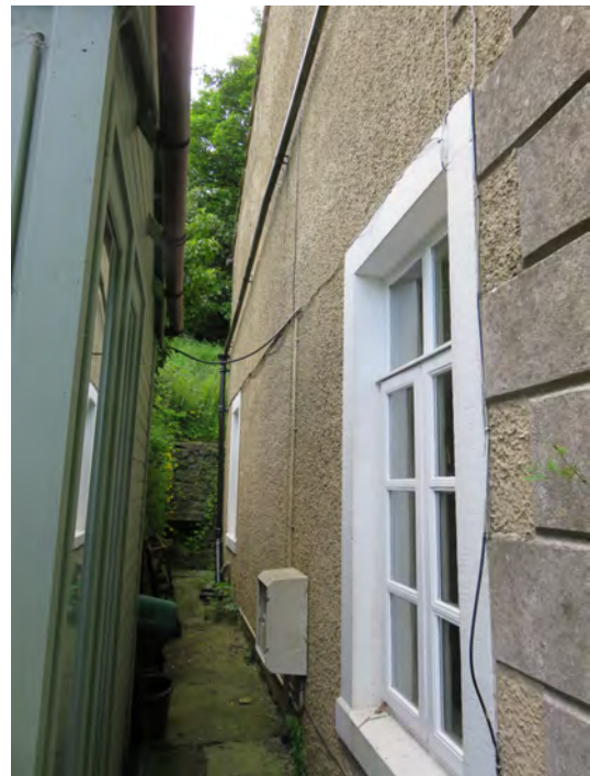
Exterior view of existing Dining Room corner window, where link through to Garden Room will be formed.
