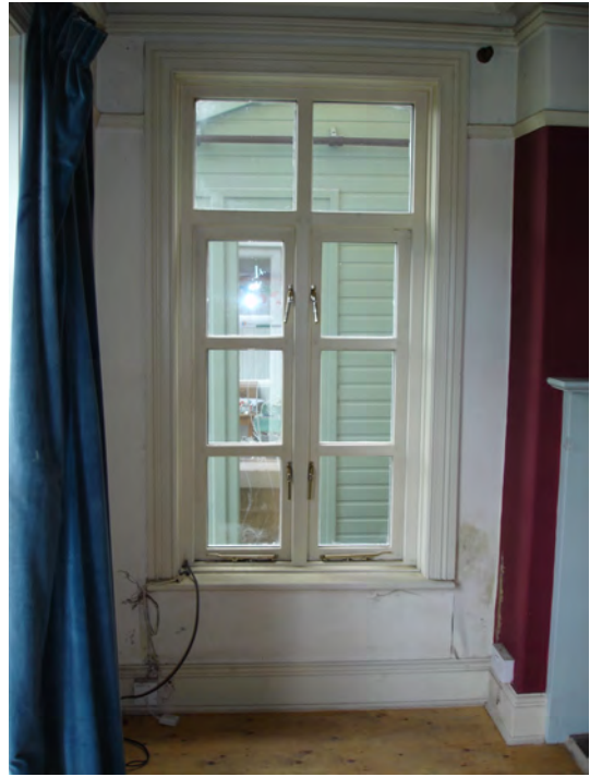
Interior view of existing Dining Room corner window, where link through to Garden Room will be formed.
