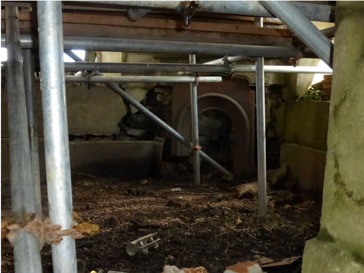
Internal Cracking on Plasterwork and Loose Stone along East Elevation
