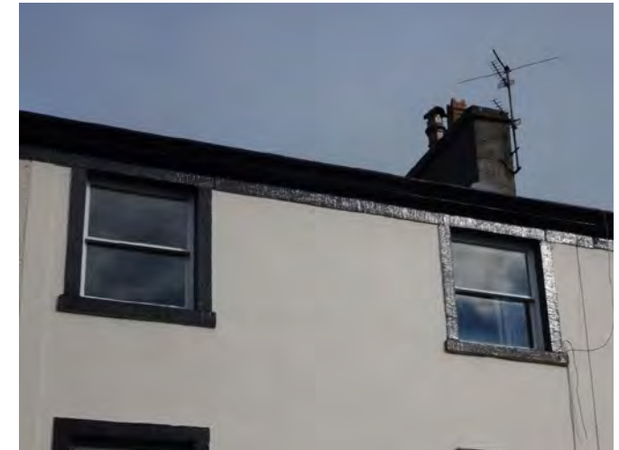
ii) Existing second floor windows to No. 17 (York Street elevation) relevant to this application.
