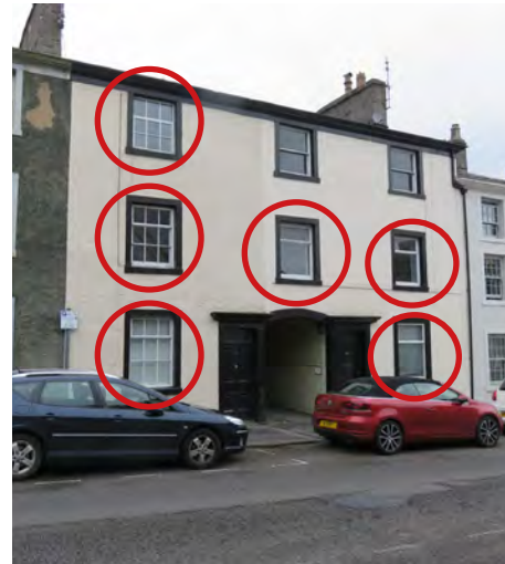
i) Front elevation to York Street with windows already granted consent for replacement shown circled.
