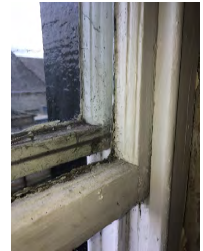
v) Internal view of window WS.2 - Second floor, No. 17, showing general condition.
