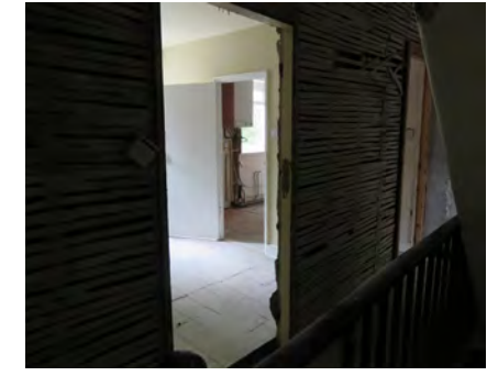
ix) Number 15 - item 11 - opening from first floor landing to rear left room.
