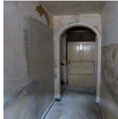
i) Number 15 - items 1 & 2 - location of former opening to front reception room and blocked doorway to rear.
