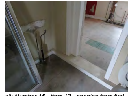
xii) Number 15 - item 13 - opening from first floor existing bathroom to rear right room.
