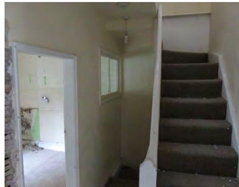
xxiv) Number 17 - items 25, 27 & 28 - glazed screen & door opening to existing kitchen and modern balustrade to stairs.
