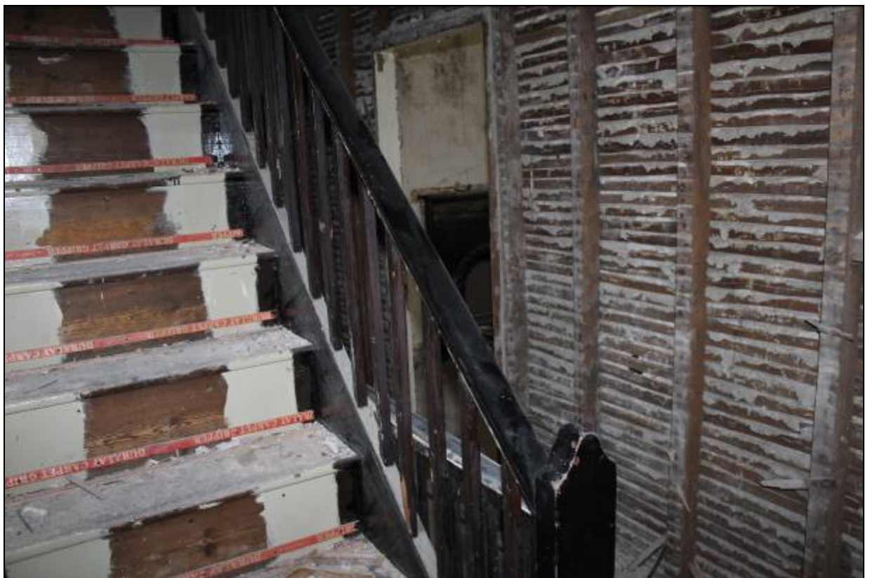
17. Staircase to second floor of 15 and lath and plaster wall of rear bedroom
