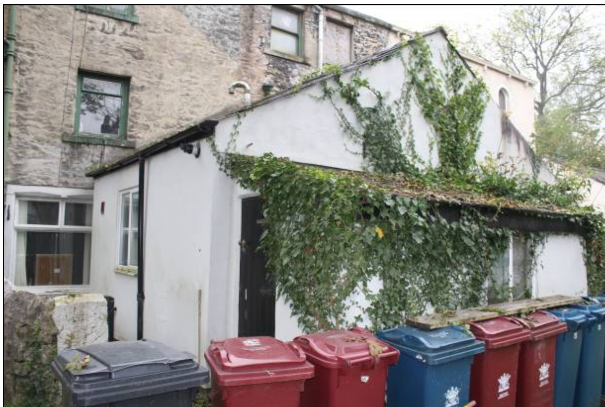
9. Outrigger of 15, rebuilt or extended by 1932 and with a further modern extension under single-pitch roof
