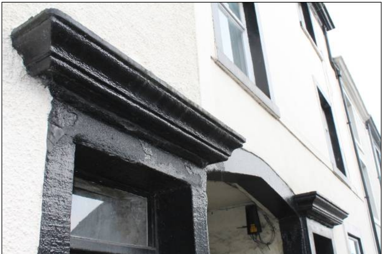
4. Doorcases with cornices in typical Regency style, suggesting a date of circa 1820-1840
