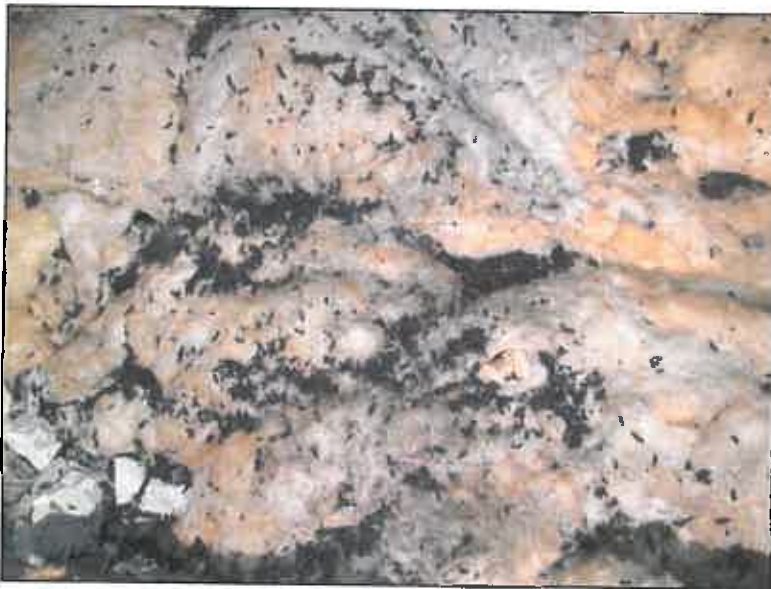
Photo 2: Accumulation of bat droppings in the building loft
