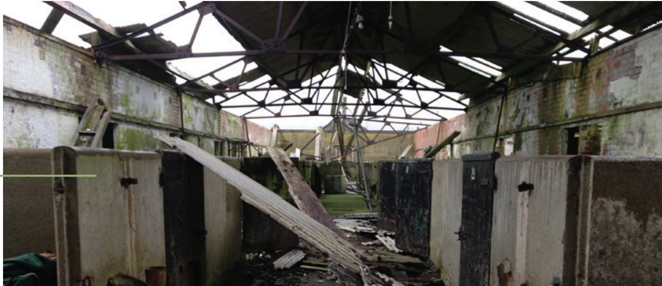
INTERNAL VIEW ILLUSTRATING POOR CONDITION AND UNSAFE NATURE OF EXISTING STRUCTURE
