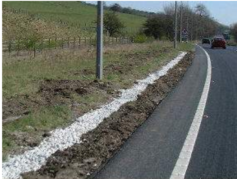
Photo showing edge of carriageway filter strip
