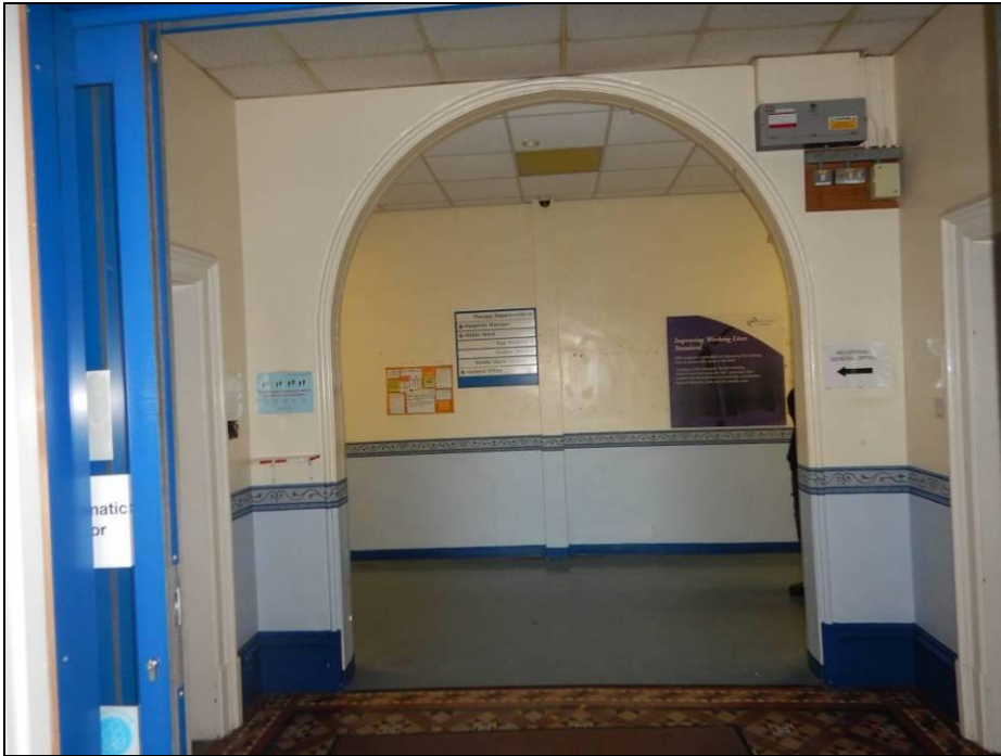
Photograph 5: An original arched opening. Some have been partially infilled and modern doors inserted.
