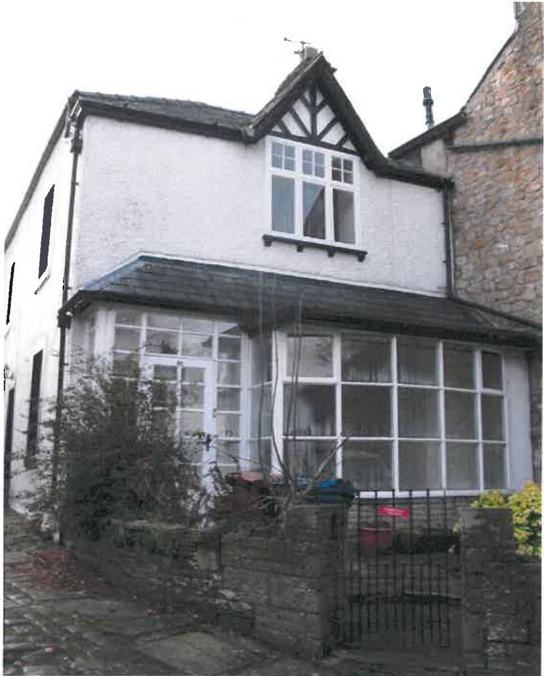
Detail of Later flat roof bay window, which projects beyond the original slate canopy roof. The bay is to be replaced with a smaller bay in keeping with the existing canopy structure.
