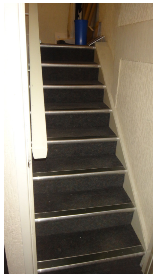
Bottom flight of stair to be replaced with new flight to extended half landing
