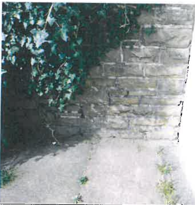
PHOTOGRAPH No. 12: SPALLING OF POINTING TO MORTAR JOINTS OF WALL FACE AT LOW LEVEL ADJACENT GABLE TO NO. 11 YORK STREET.
