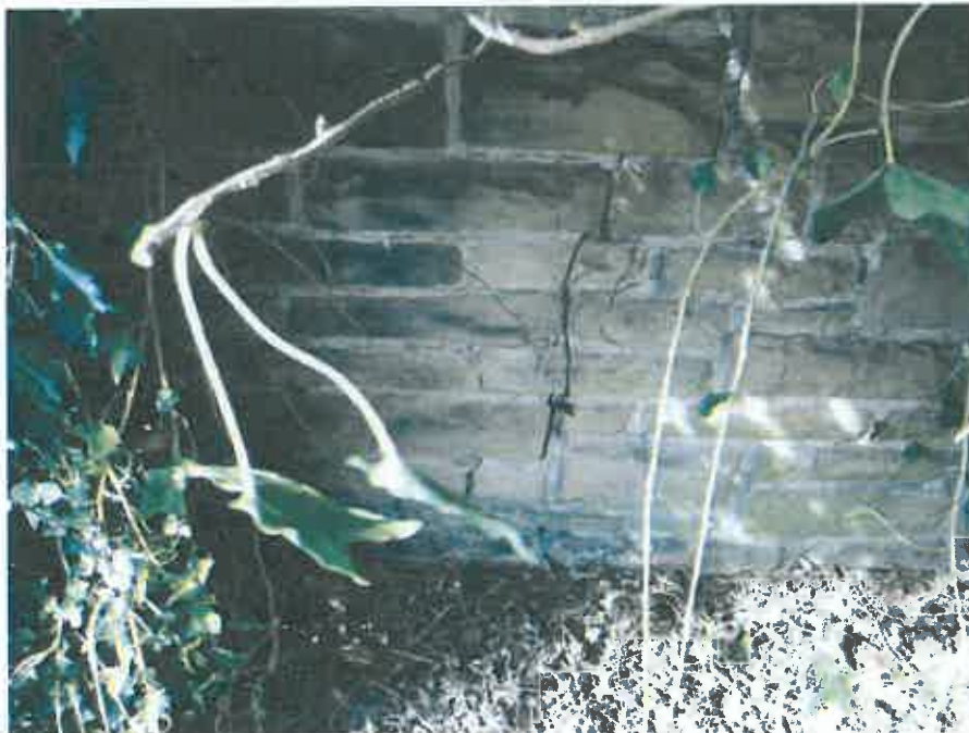
PHOTOGRAPH No. 10: 3MM-5MM WIDE STEPPED VERTICAL CRACK EXTENDING OVER FULL HEIGHT OF FRONT WALL FACE IMMEDIATELY IN FRONT OF EXISTING TREE. CRACK EXTENDS ACROSS STONE BLOCKS AND WALL IS DISPLACED ACROSS CRACK LINE.
