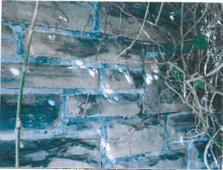
PHOTOGRAPH No. 11: VARYING HAIRLINE TO 3MM HORIZONTAL CRACK TO BELOW HEAD OF WALL AT MID SECTION OF WALL ADJACENT EXISTING TREE.
