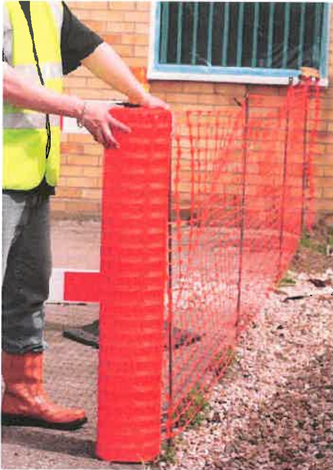
Appendix 5a: Fencing to mark out the construction exclusion zone as an alternative to heras style fencing.
