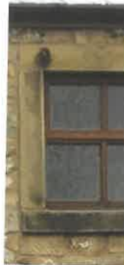
STONE JAMBS LINTOL CILL WINDOW DESIGN FRAMES CROSS SECTI MATCH THAT AS EXIST
