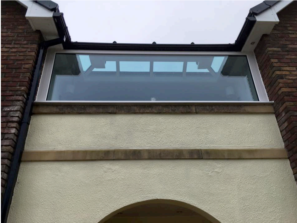
Photo 3: Glazed panel installed above render wall detail to enclose previously open front balcony Area (As implemented, external view)
