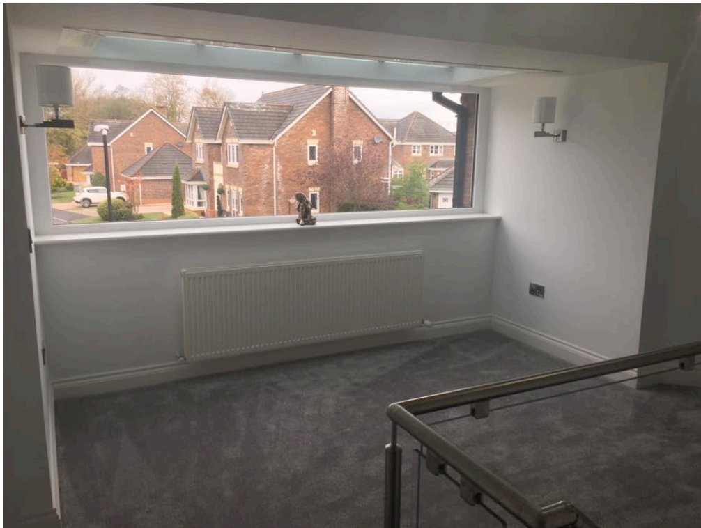
Photo 4: Glazed panel installed above render wall detail to enclose previously open front balcony Area (As implemented, internal view)
