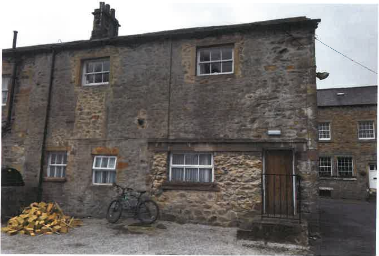
PL16 showing the rear elevation of the west area of the building. The once existing entrance to the garage and possibly even the stables can clearly be identified through the area of infill to the right at ground floor level with the stone head / lintel located above.
