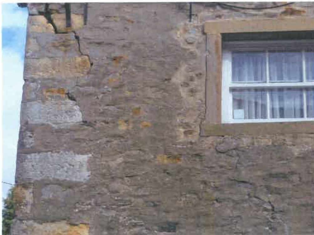
Front Elevation – cracking
