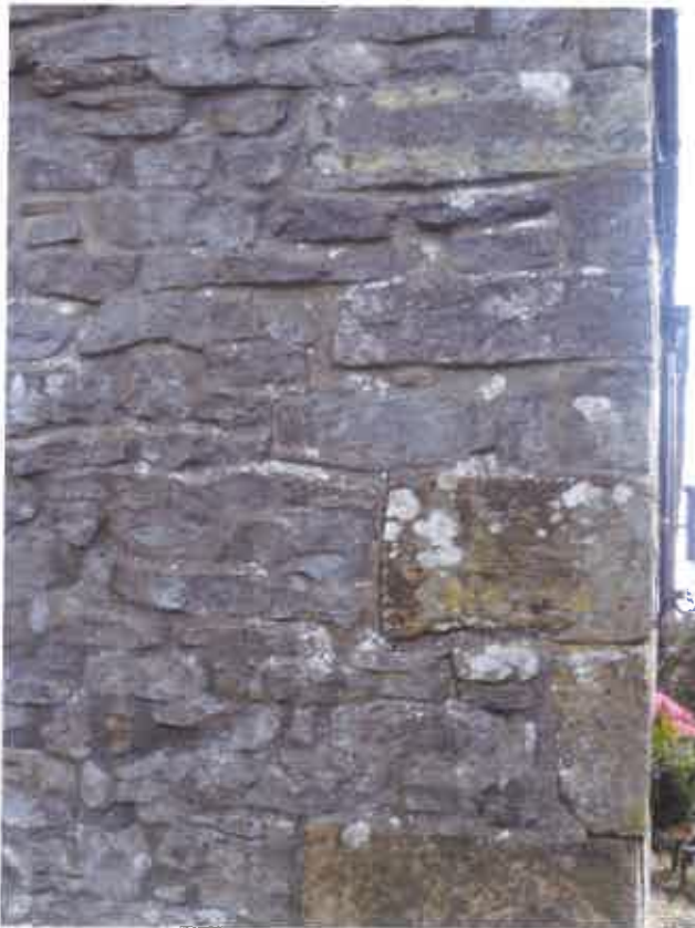
Left Hand Elevation – cracking
