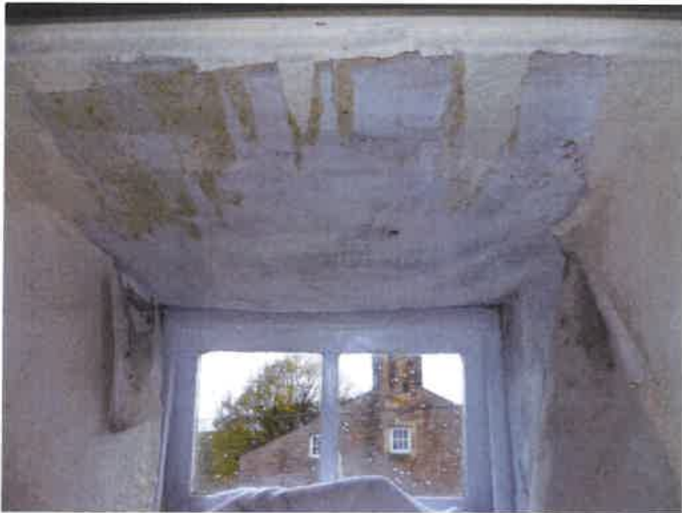
Gable window – water penetration
