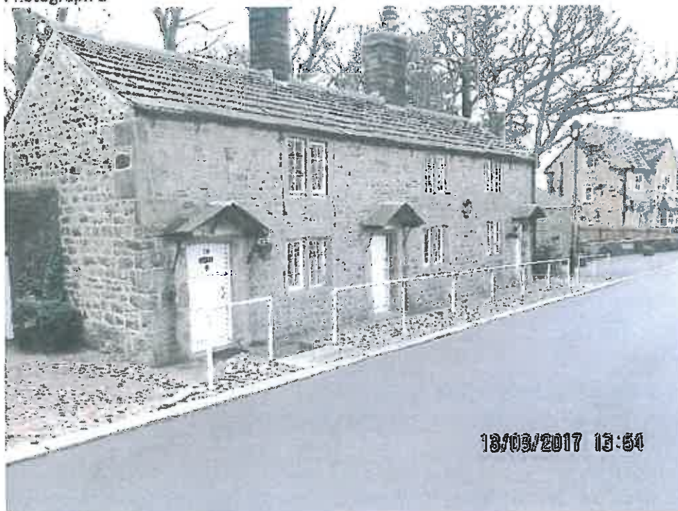
John Brabyns Alms houses, stone slates, cast iron guttering (large quoin stones), random stone courses, mullion stone surrounds with Georgian windows, circa 17 th century, Grade II
