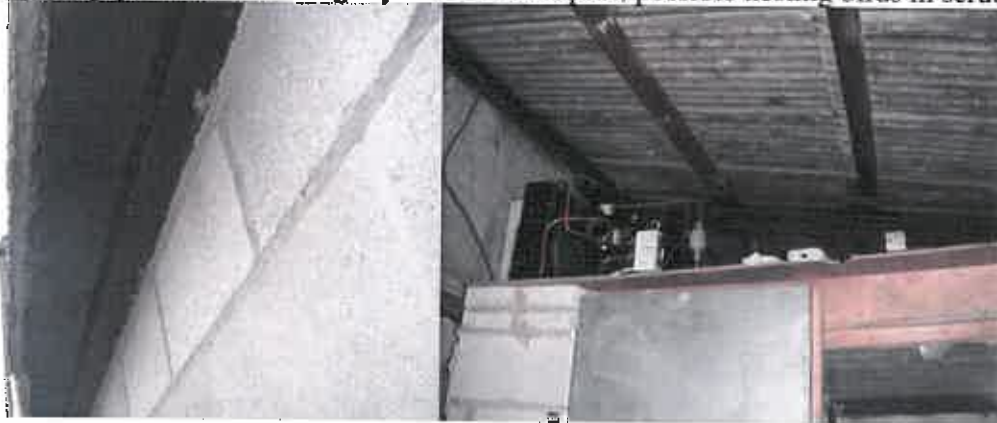
P3 Gap under lintel, but not suitable for bats P4 Inside showing unlined corrugated roof
