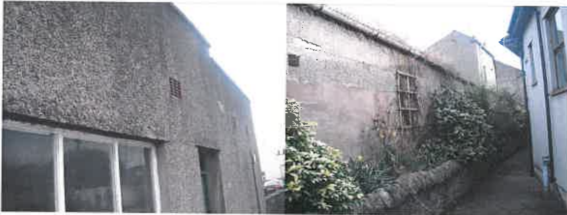
P1 Front aspect, gaps in vent, but brightly lit P2 Rear aspect, possible nesting birds in scrub
