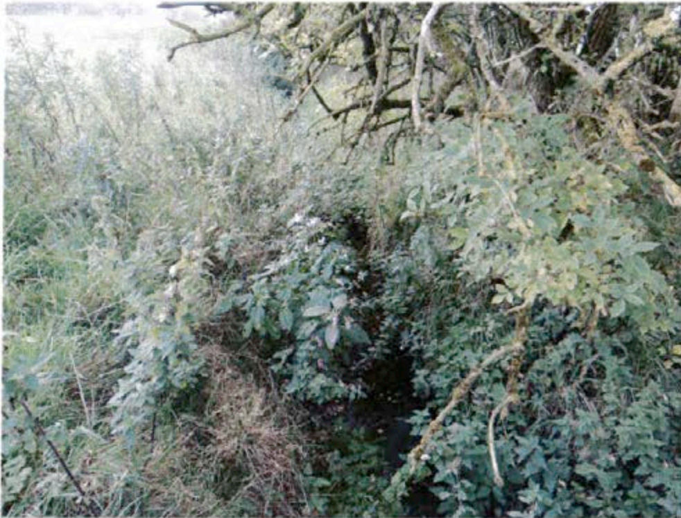
Fig (iii) : Overgrown ditch on eastern boundary.
