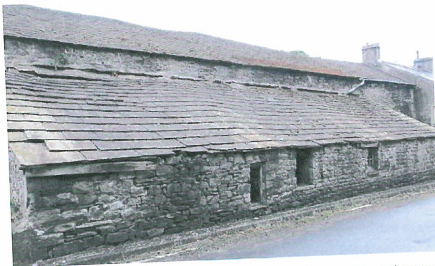
Photograph (4) – North elevation Stones missing north east corner
