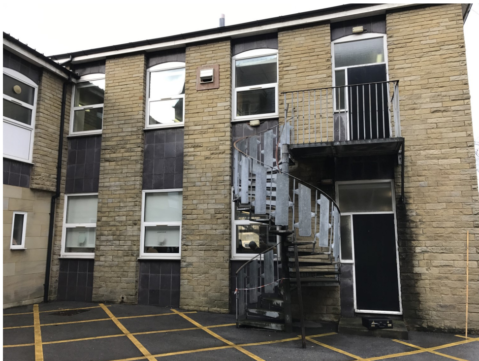
View of the existing damaged staircase
