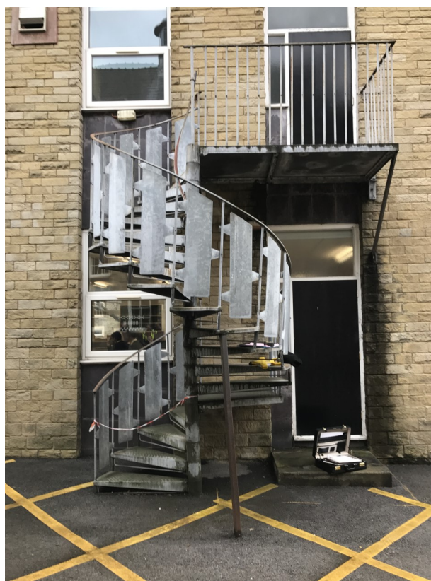
View of damaged spiral staircase
