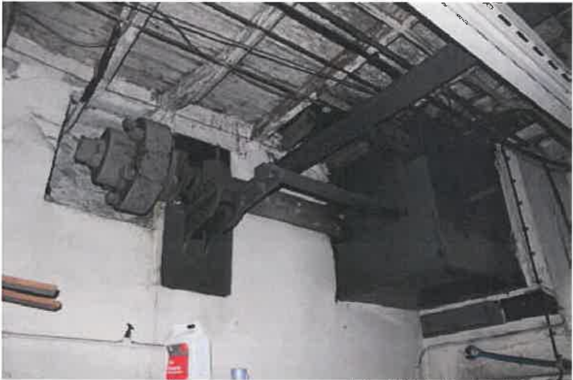
Plate 57: Enclosed bevel gear on secondary motion shaft, with further bearing to left
