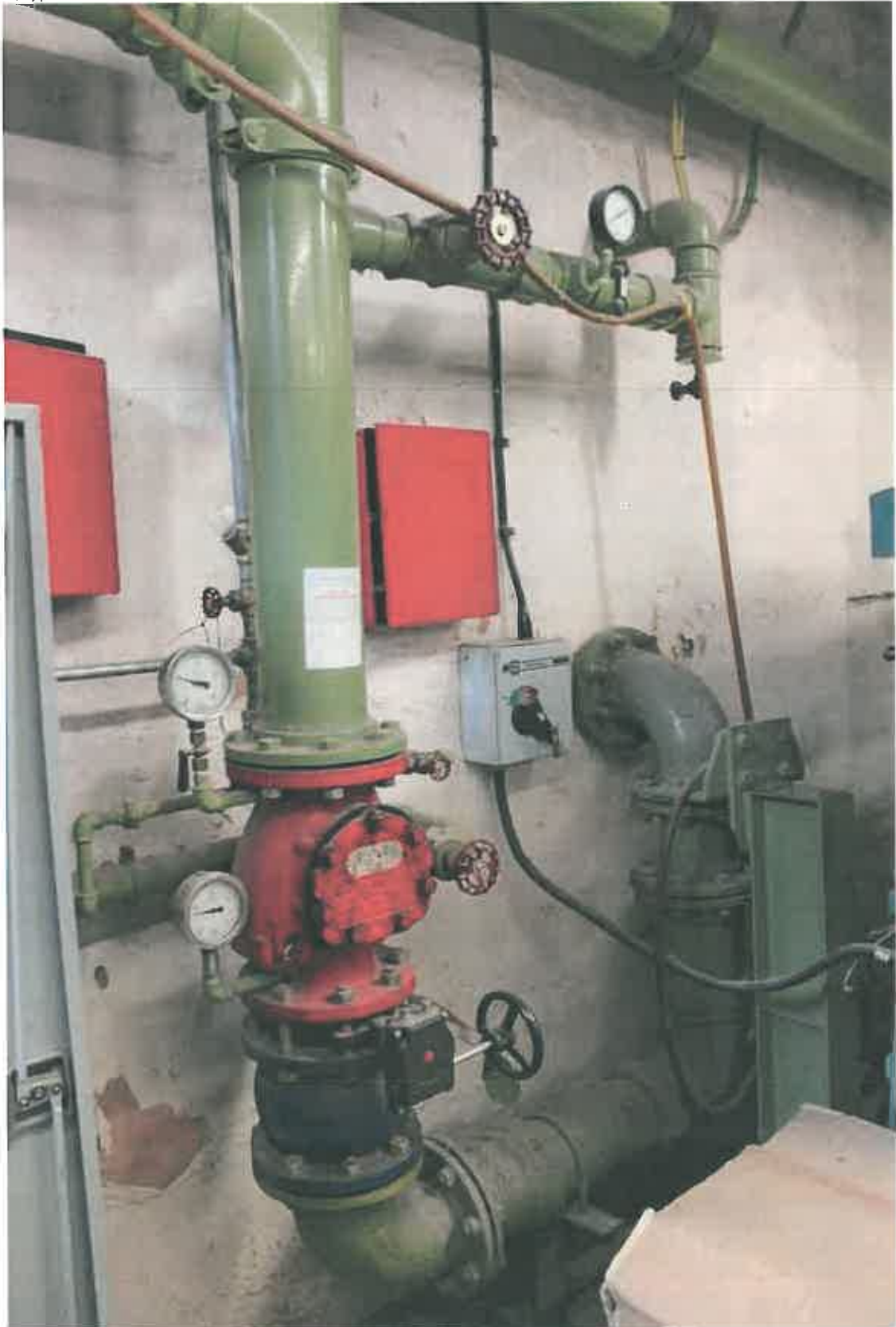
Plate 75: 'Christmas Tree' control valve for New Mill automated sprinkler system
