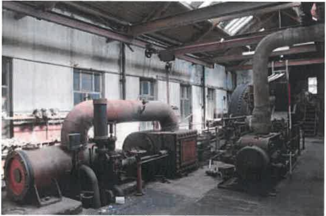
Plate 99: View of the engine, looking north-east
