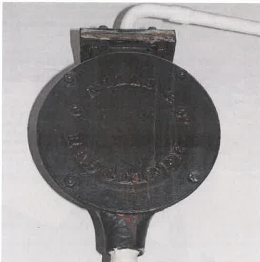
Plate 76: Pressure valve in sprinkler system, bearing maker's stamp
