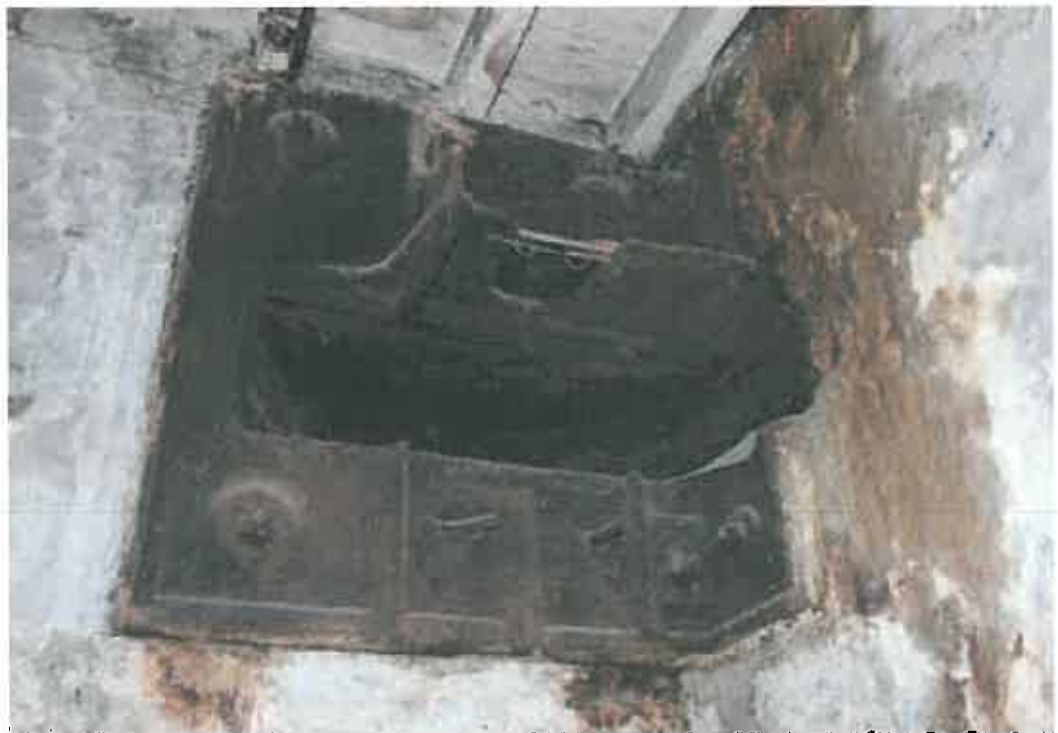
Plate 72: Upright shaft top end bearing, second floor, New Mill
