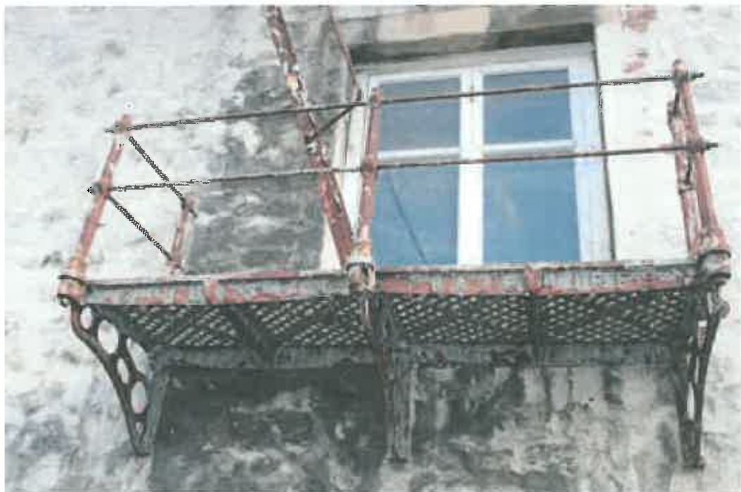
Plate 73: Maker's stamp on external fire escape landing
