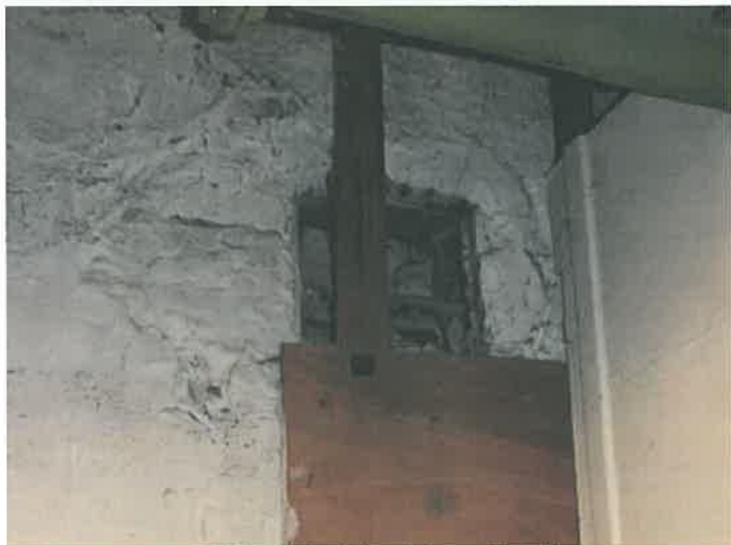
Plate 63: End bearing box for line shaft, ground floor, New Mill
