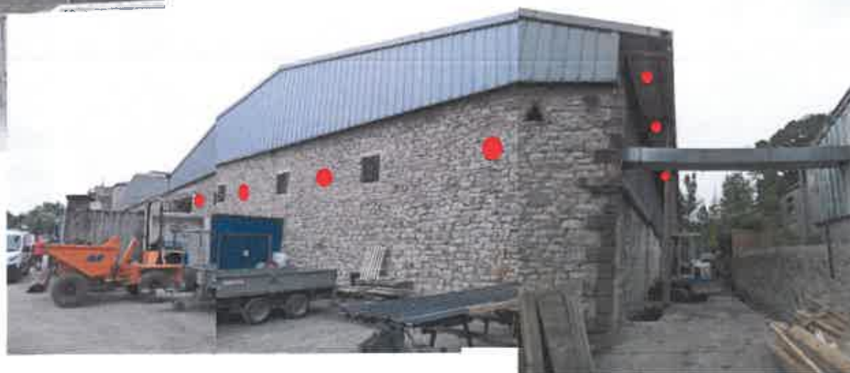
LED Floods Under Eaves
