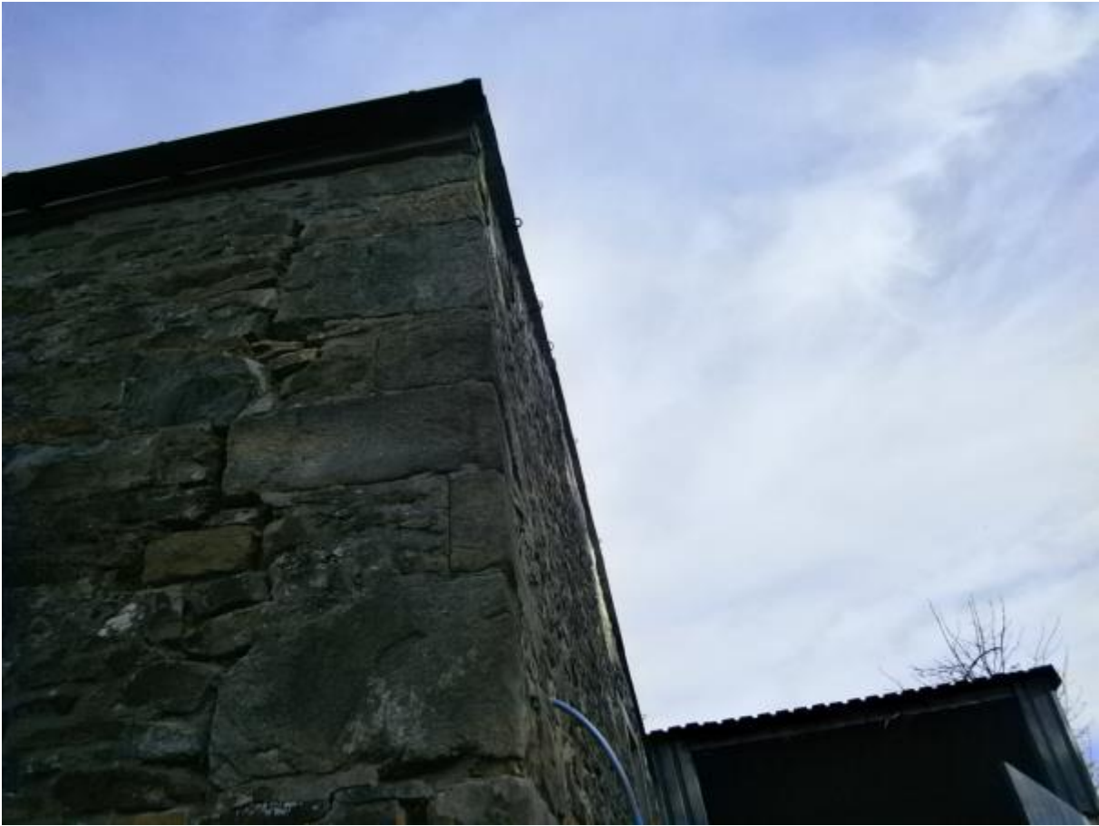
Photo 22 - South East Elevation- indicating bow inwards
