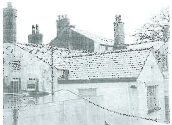
Target Note 4: Rear elevation of pub with moderate - high bat roost potential due to various roof access points.
