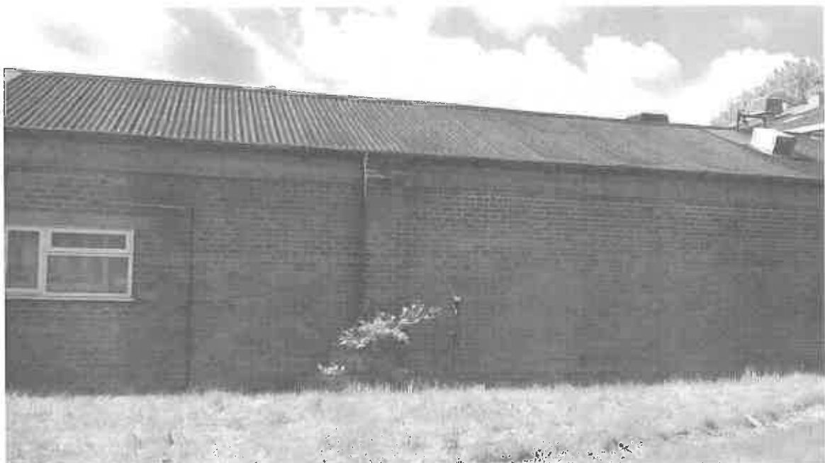
External monitoring location No2 Midway between extraction filter unit and monitoring location No1
