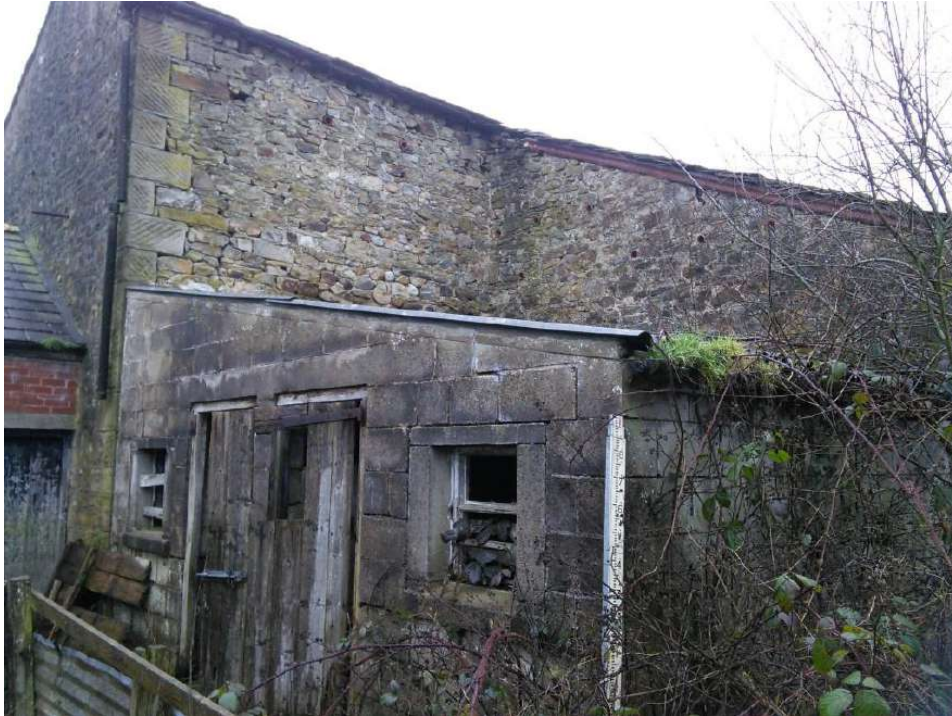
Figure 11 The south-east elevation of Barn One showing the modern lean to structure
