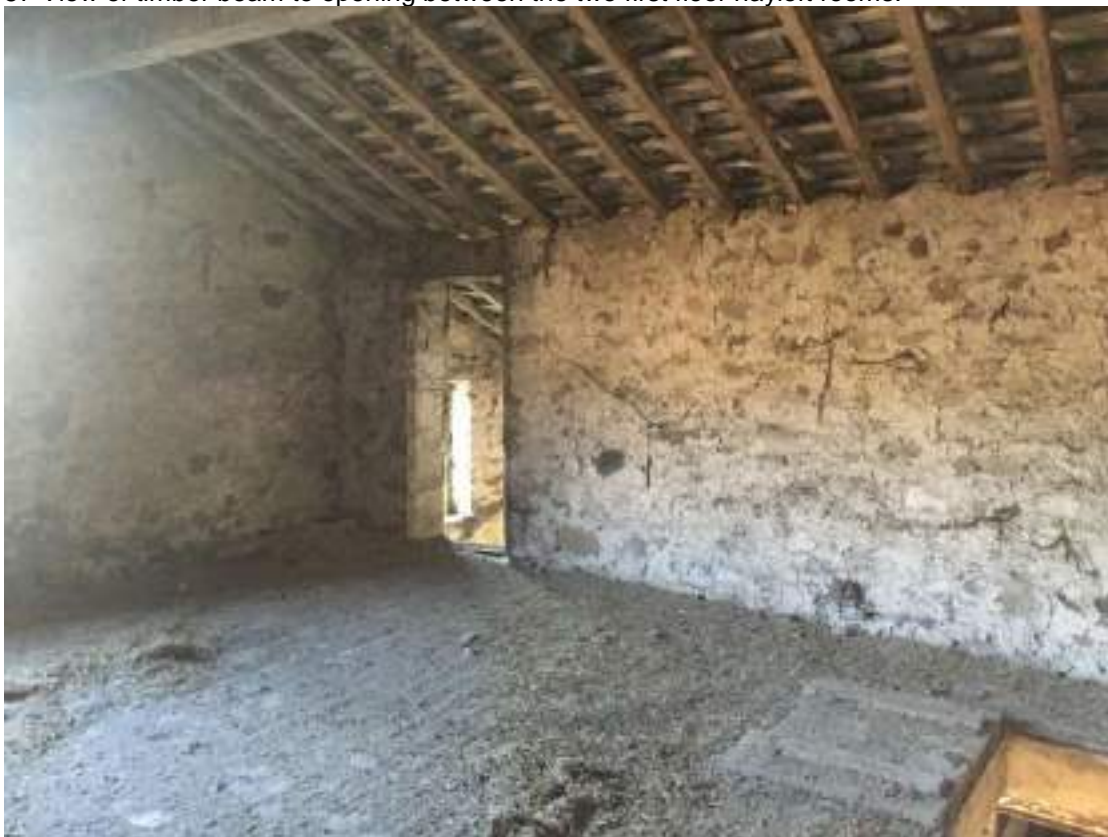
58 View towards southeast elevation showing opening to rear outshut and access hatch.
