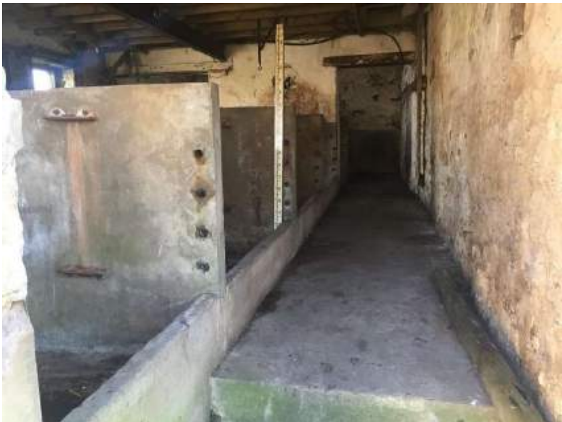
44 View into large shippon showing concrete cattle stalls and raised concrete floor, note low level concrete upstand and holes in stalls where steel tubing has been removed.
