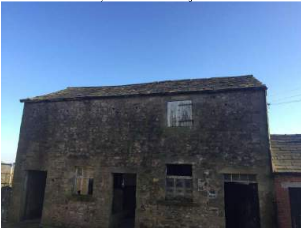
6 Front elevation of the two-storey barn showing ground and first floor openings, note stone flags to main barn roof.
