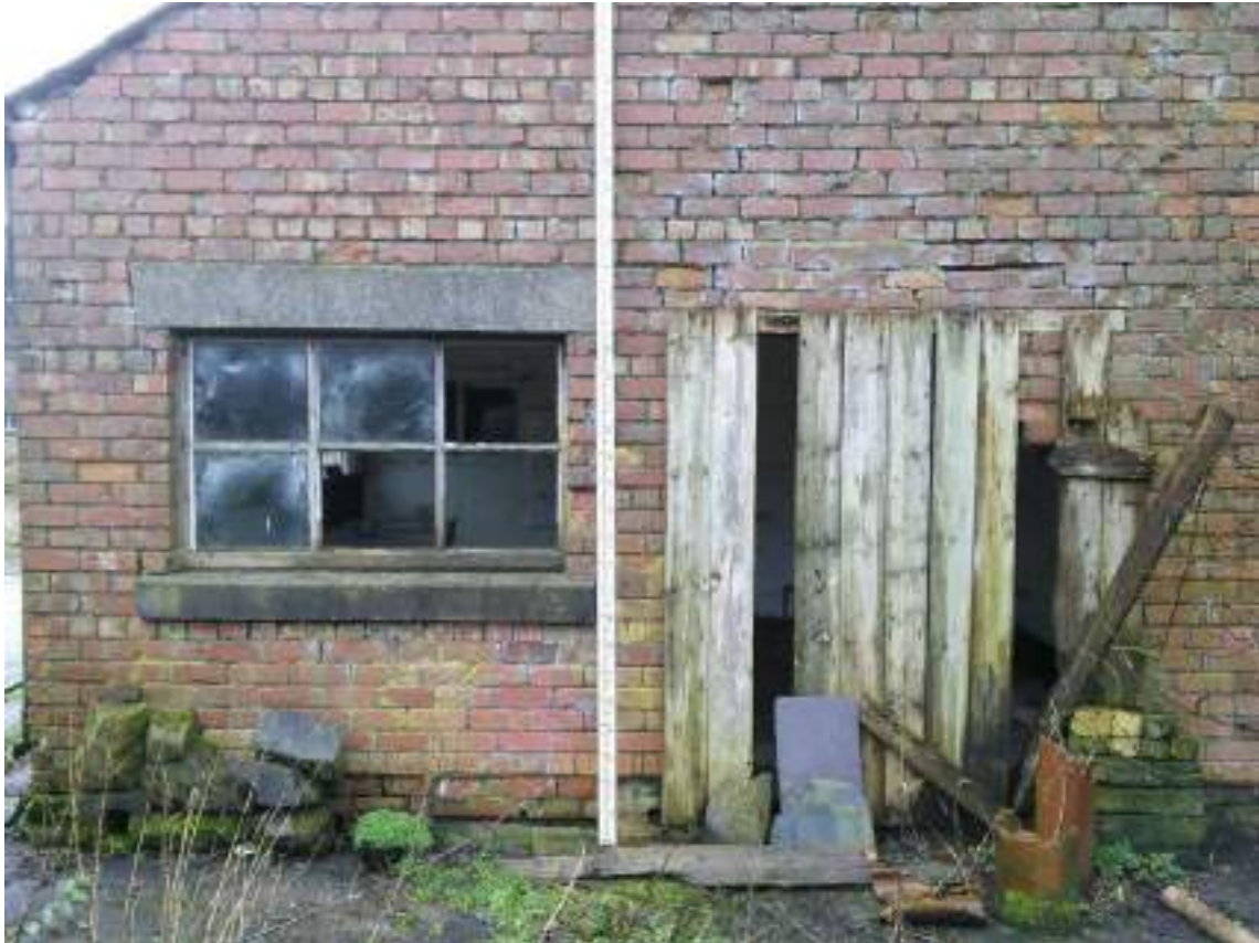
29 Window and door detail, note spalled brickwork and damage to door opening.
