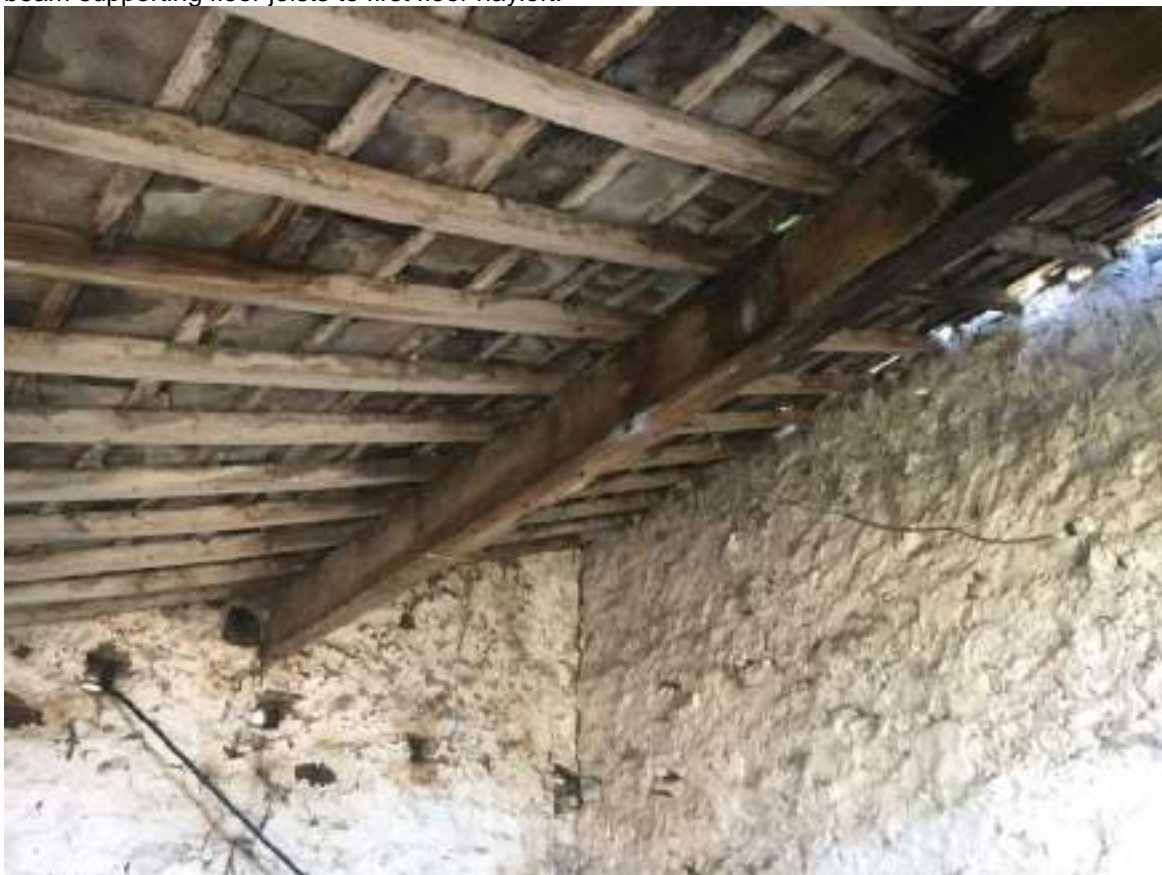
48 View of timber roof to rear shutout showing purlin spanning between gables supporting rafters.
