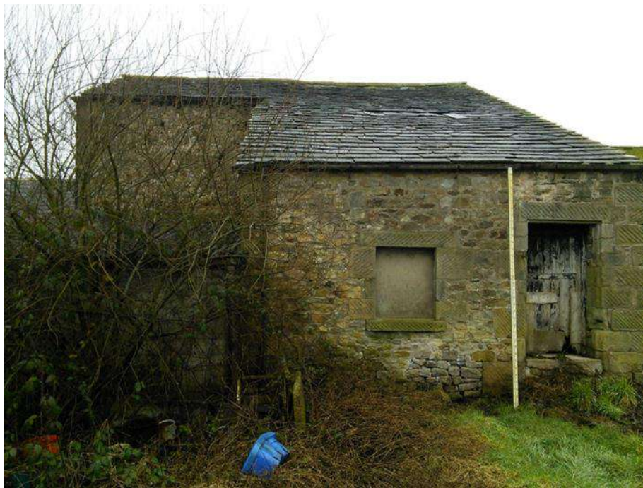
Figure 10 The south-east elevation of Barn One showing the rear outshut structure and disused slurry pit outside rear doorway.
