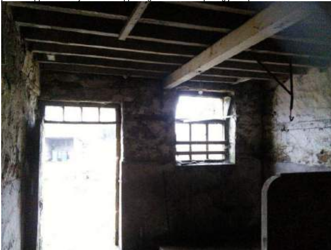
40 View of front wall showing fanlight over door, floor joists and supporting timber beam.
