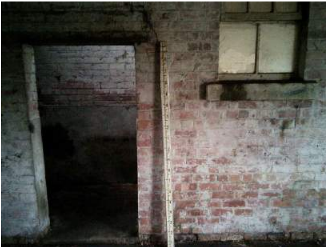
36 Internal view of store room showing internal window. This was possibly the external wall prior to the gap between the two structures being enclosed; RH wall.
