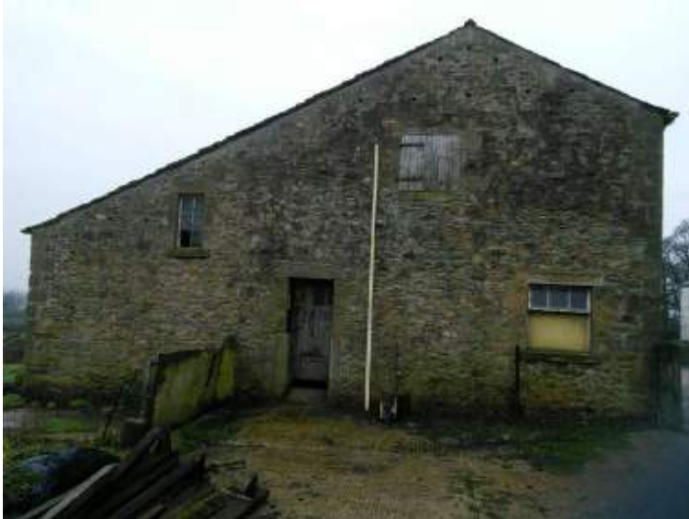
13 Left Side (north east) elevation of the two-storey barn with extended shutout and side access door for cattle
