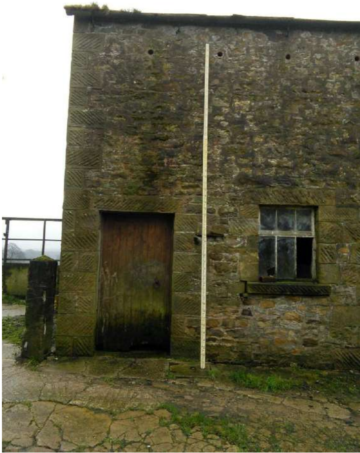
11 North west entrance door leading to shippon, note ventilation holes at first floor level for cross ventilation of hayloft at first floor
