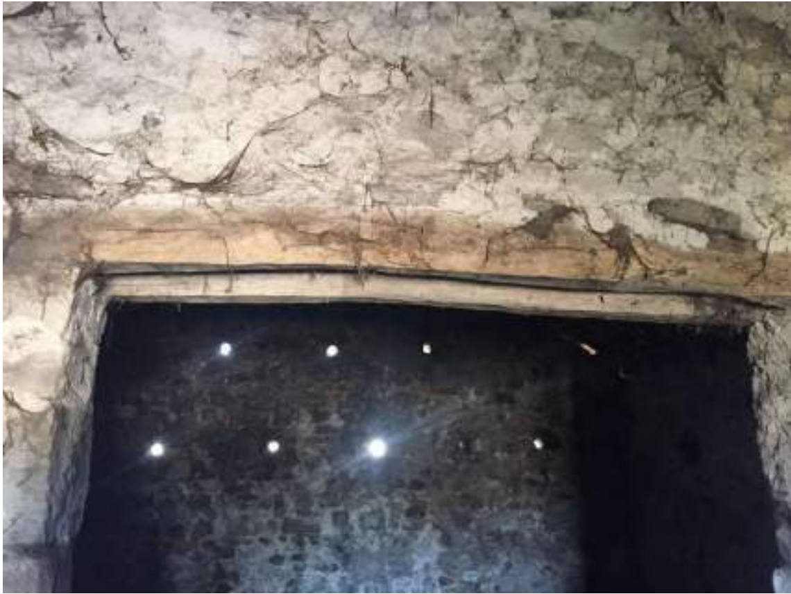
57 View of timber beam to opening between the two first floor hayloft rooms.
