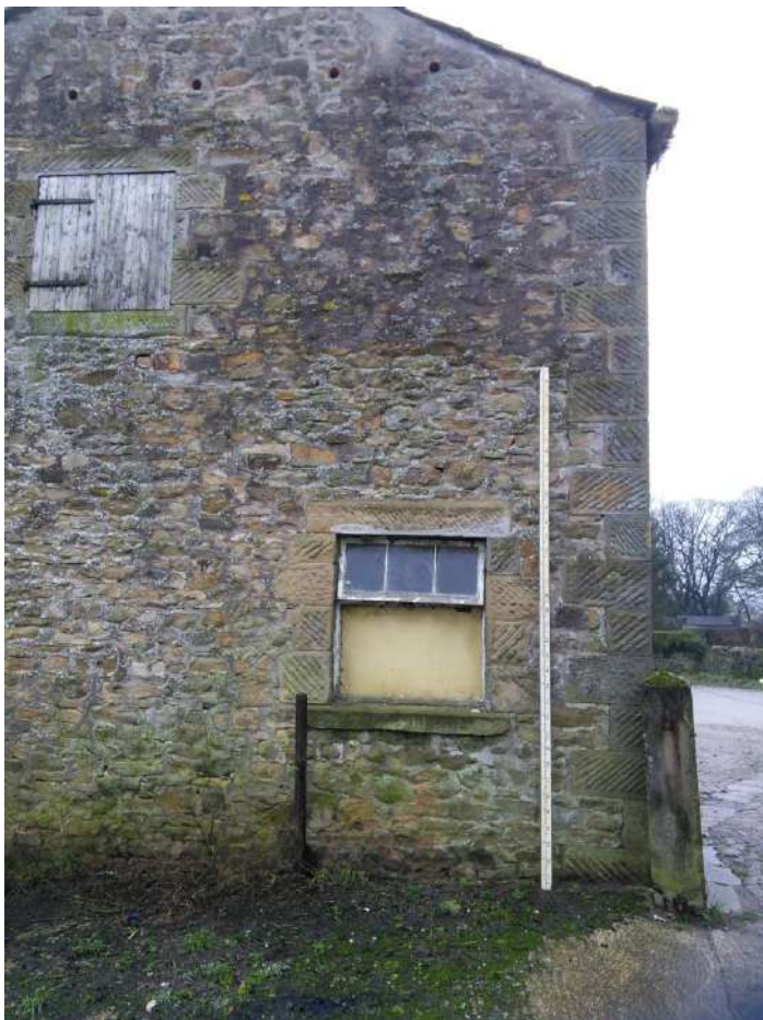
14 Detail of corner stone quins and openings. Note first floor door directly hinged to stone quins.
