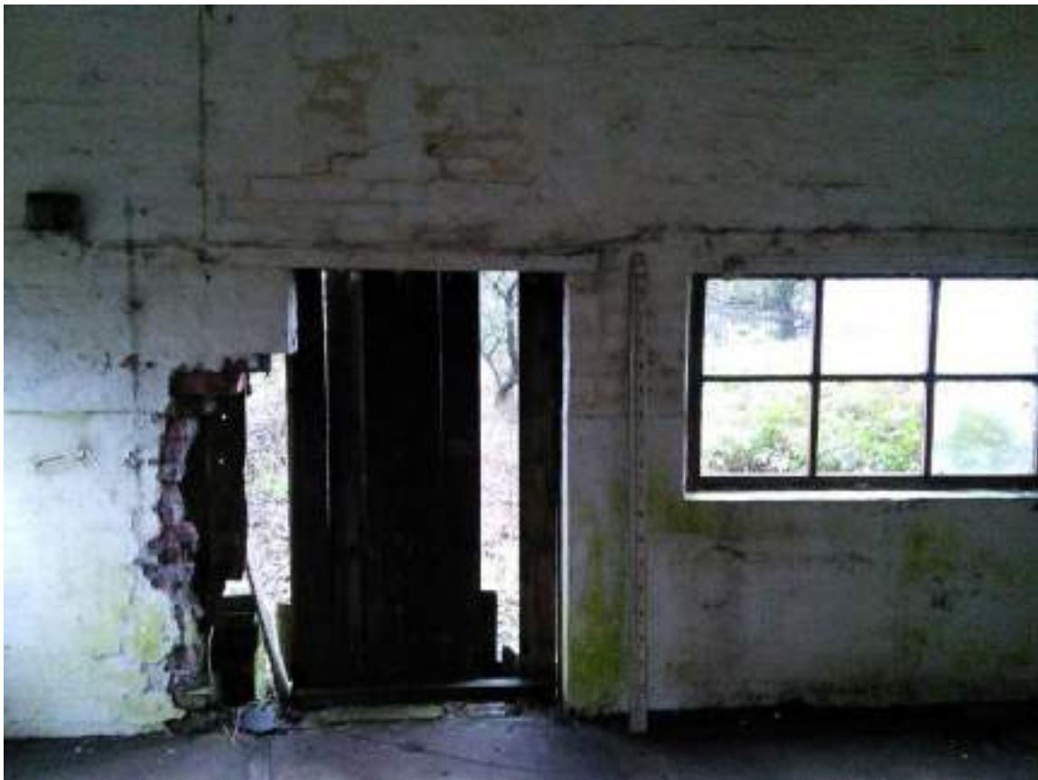
32 View showing damage to existing opening and cracking above doorway; RH wall.
