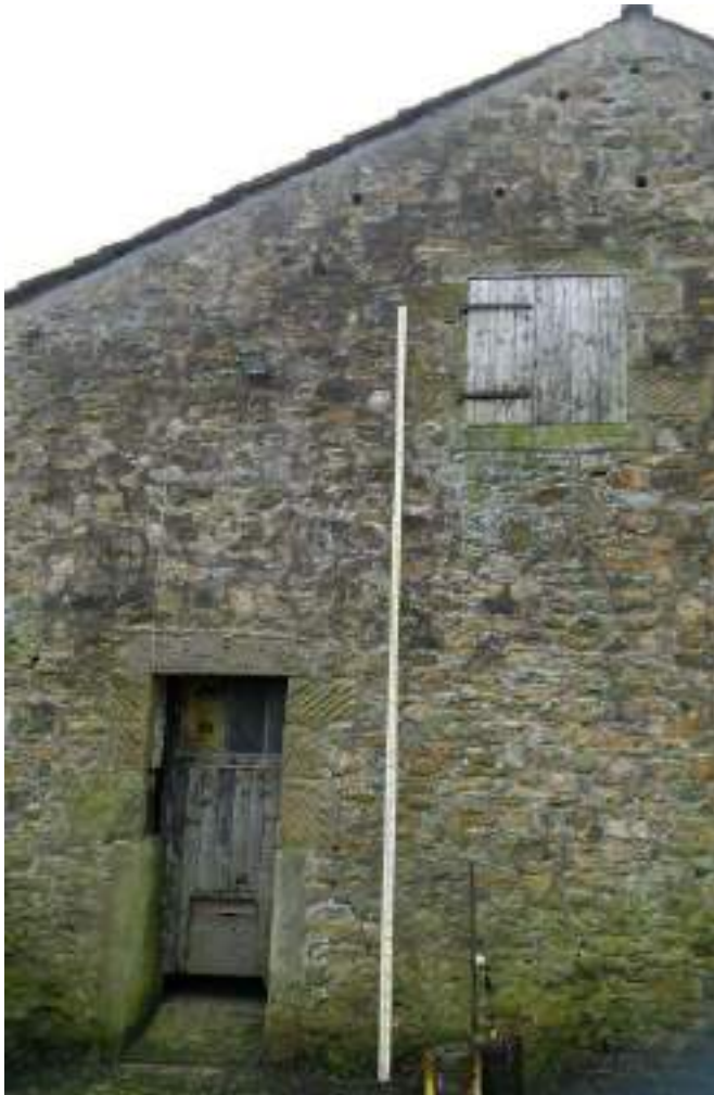
15 Detail of openings. Note ramp to access door and ventilation holes in gable.
