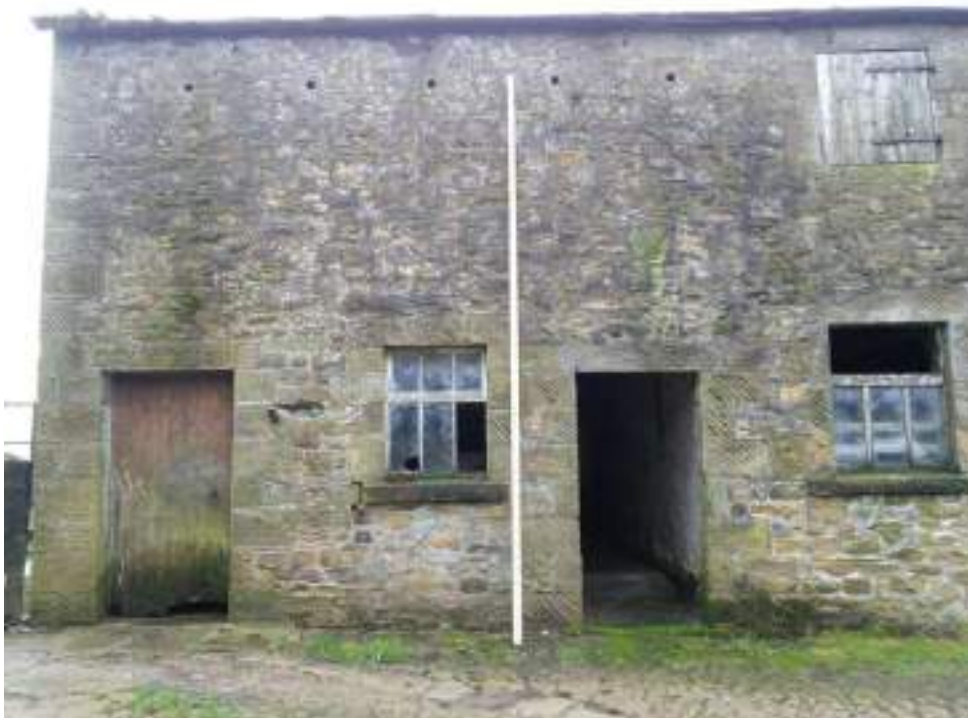
10 Part view of front elevation showing openings and ventilation holes at first floor.
