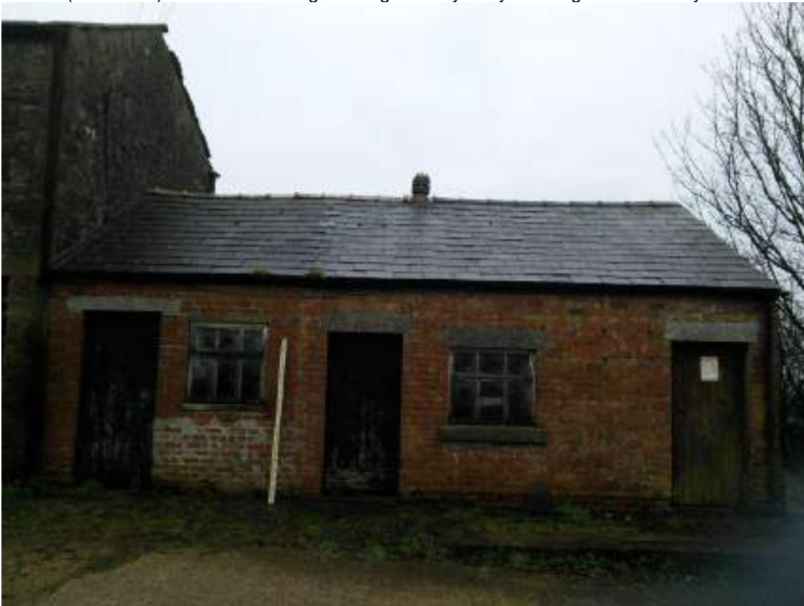
2 Front elevation of the single storey brick dairy structure with slate roof
