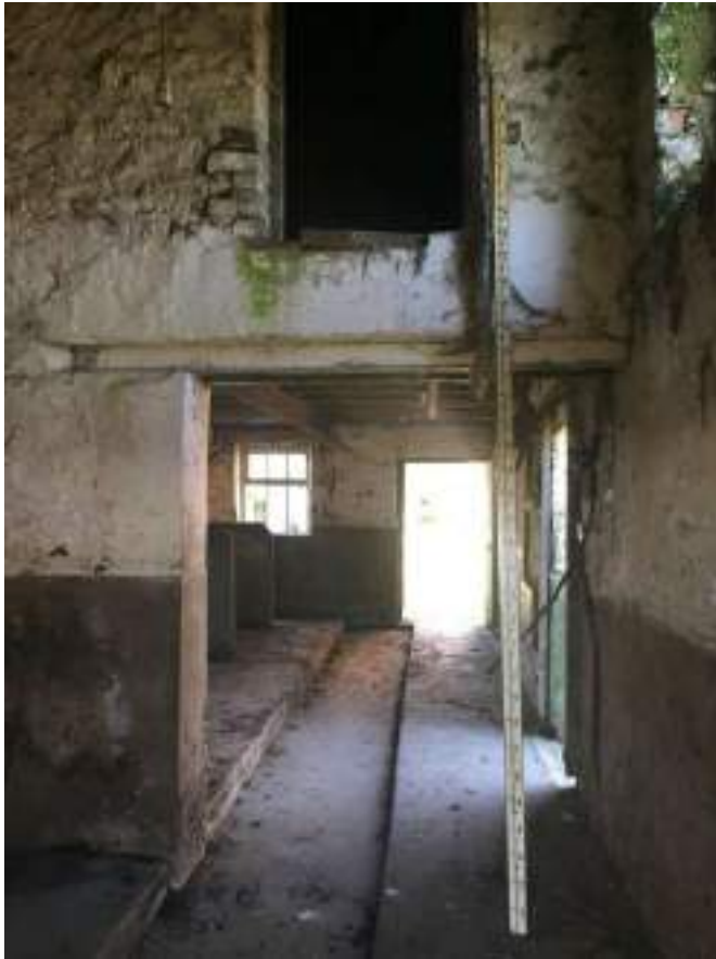
49 Internal view looking through from rear shut out showing opening. Note steel beam supporting floor in main shippon area and first floor opening.
