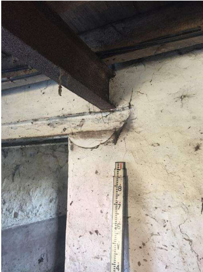
47 Detail of steel beam over opening separating main room and rear shippon and main supporting steel beam supporting floor joists to first floor hayloft.
