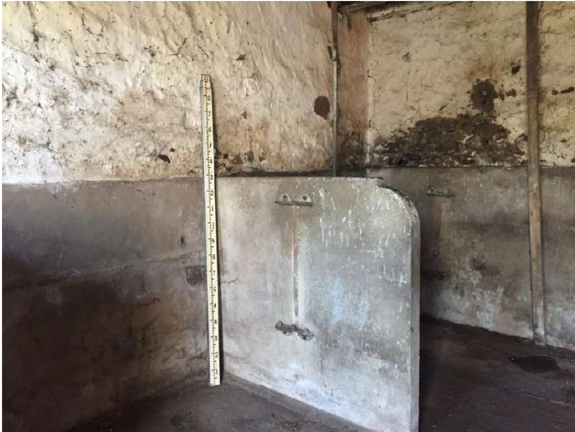
39 View into small shippon showing concrete cattle stalls, part rendered walls, concrete floor, and floor joists to upper floor hayloft. Note supporting timber beam splitting joist span.
