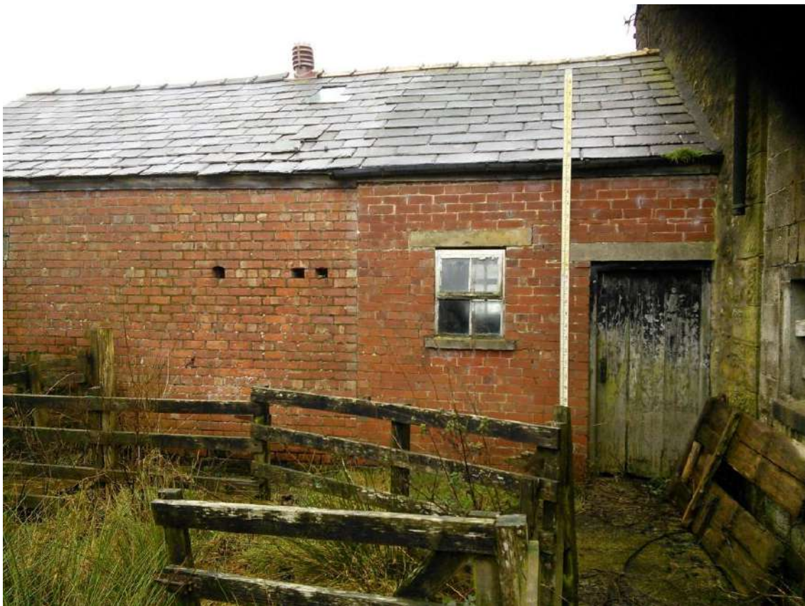
24 Rear elevation to single storey dairy building showing infill area in differing brick.
