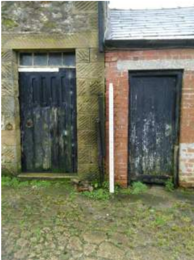
3 Junction of single storey structure and original barn showing quoins around doorway and timber doors
