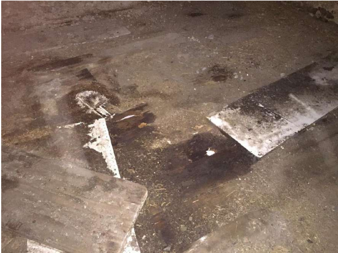
55 Water damage to floor causing rot within floor timbers.
