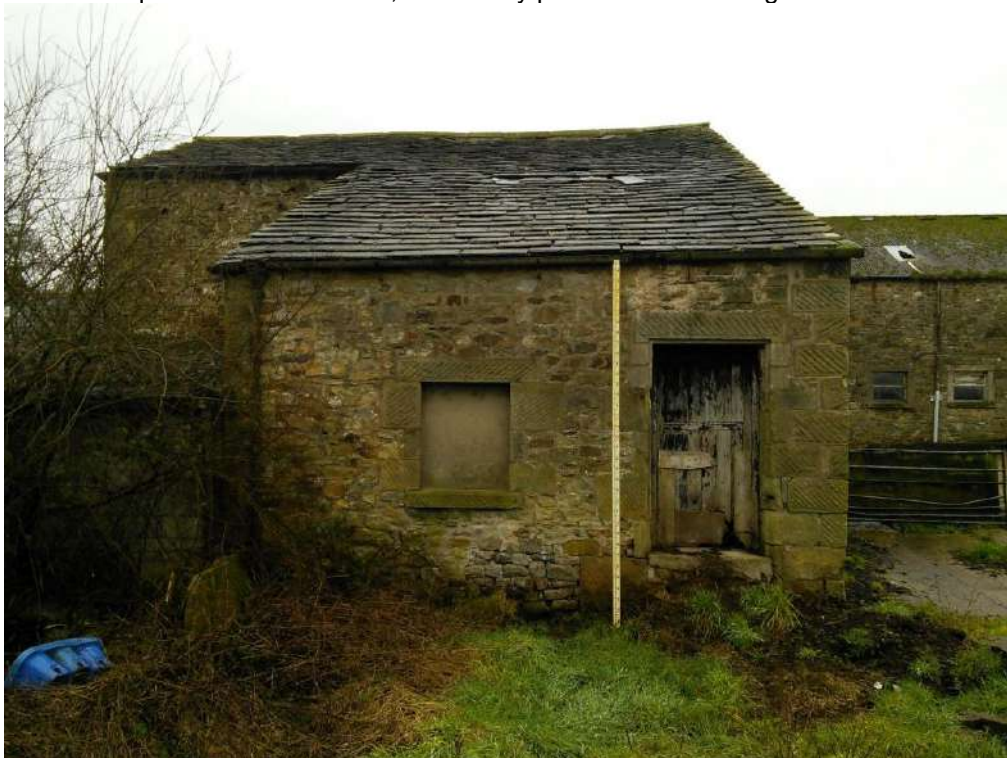
20 Rear (south east) elevation showing drop from rear door to slurry pit level.
