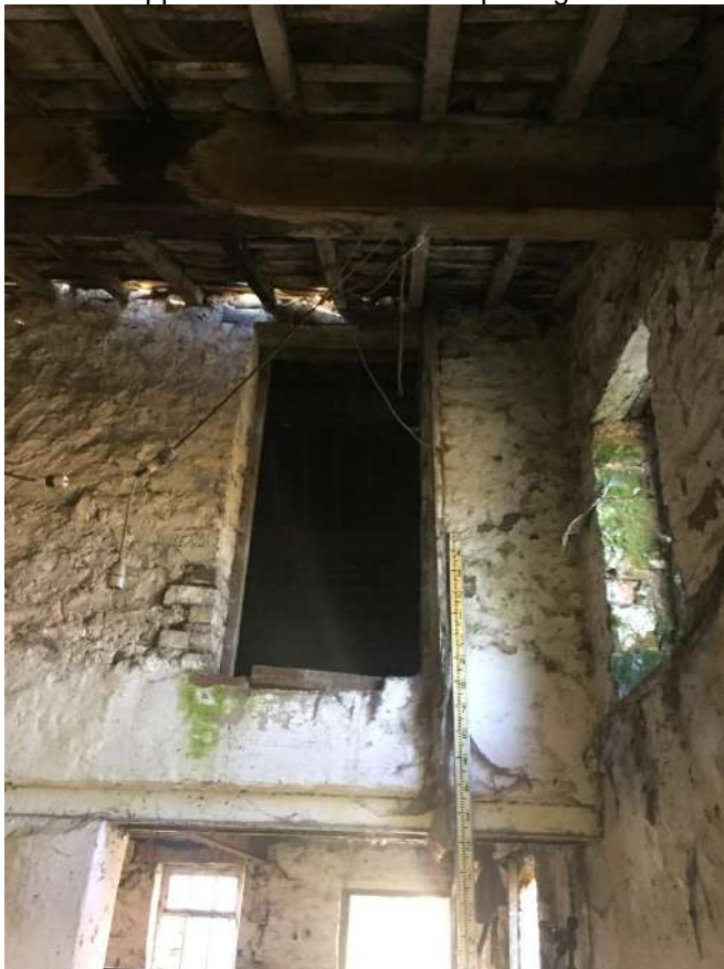
50 View of first floor opening and high level window to rear shutout.
