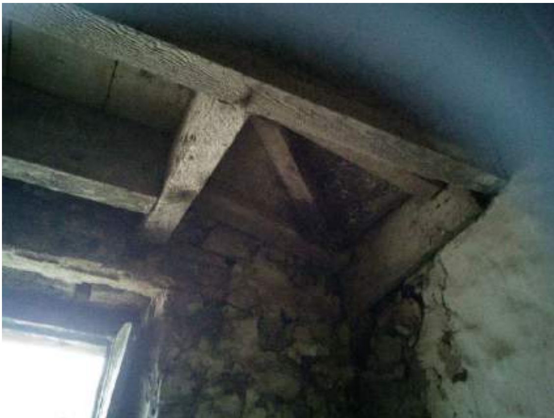
42 Trap door to north west corner of small shippon providing access to first floor.
