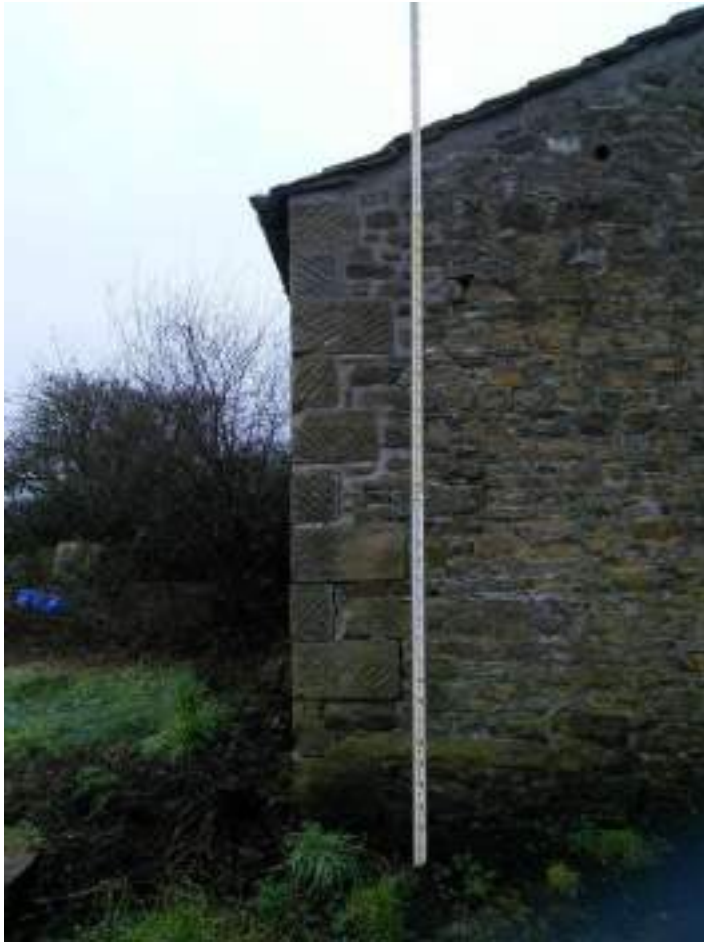
19 Corner quoin detail to outshut, note slurry pit to rear of building.
