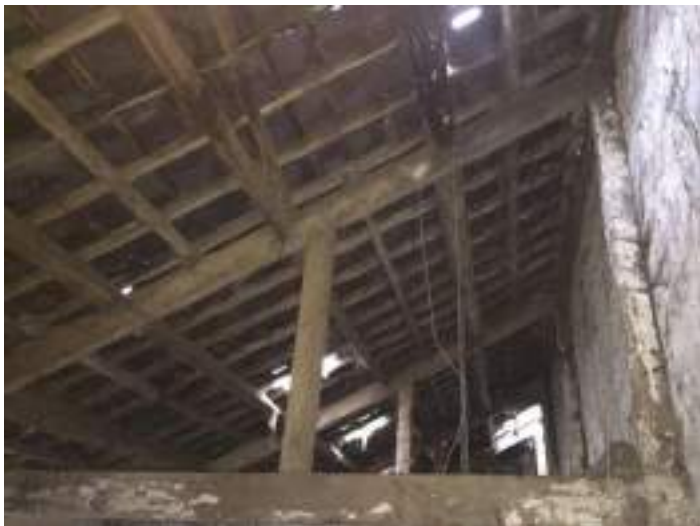
Figure 26 View of roof structure to rear outshut, note primary and secondary purlins.
