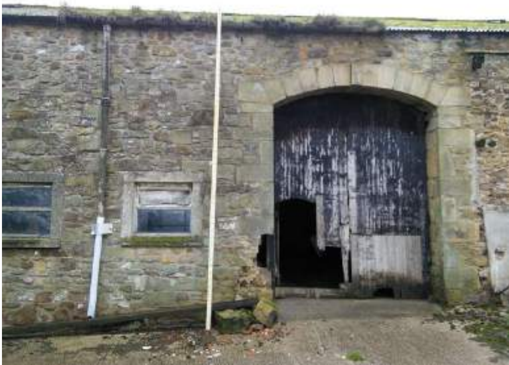
4 Stone archway to cart entrance with side quoins, note damage to bottom right hand corner
