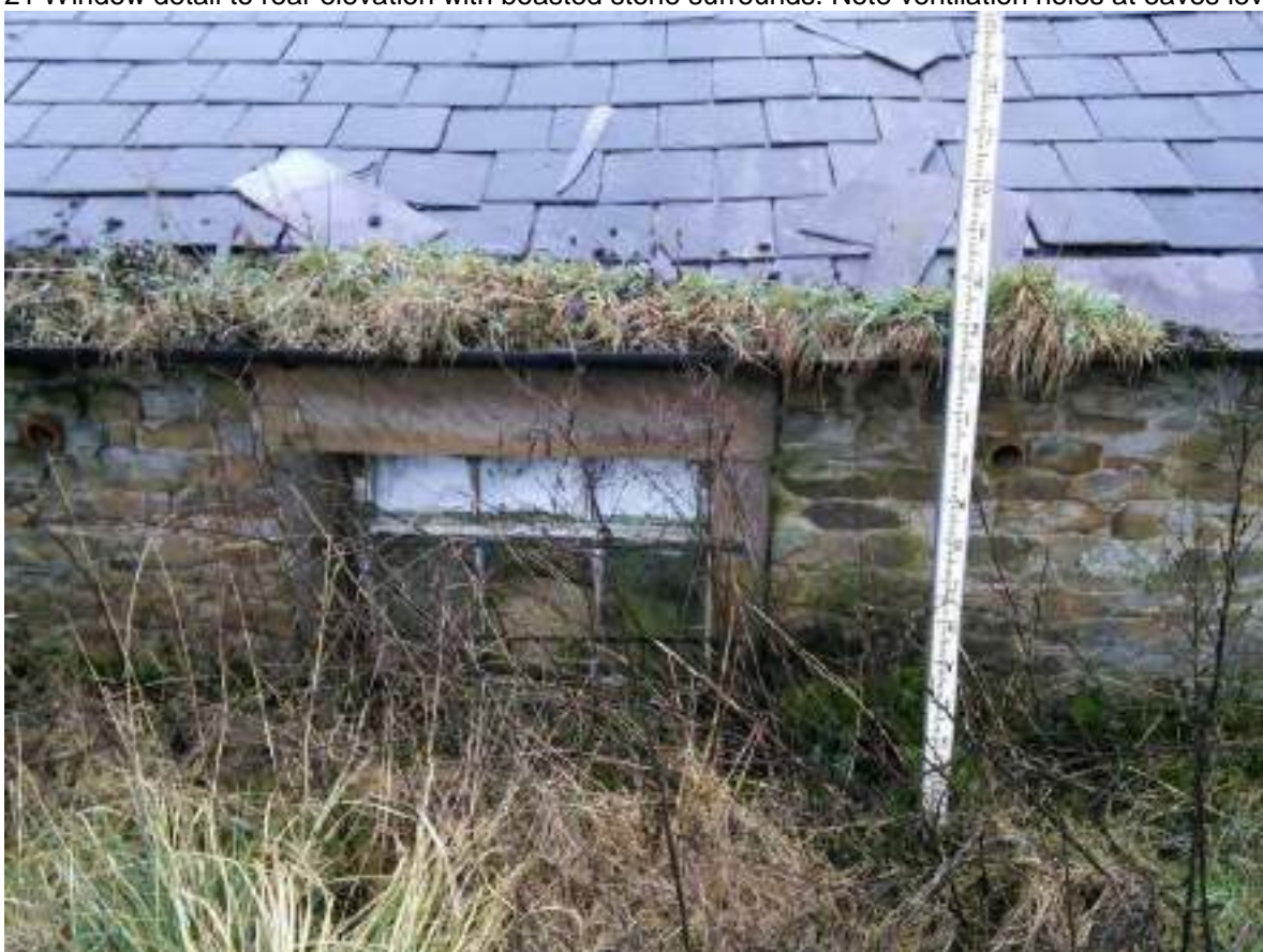
22 Left hand side window of rear elevation, note modern slate roof tiles.
