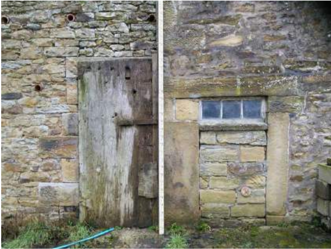
15 View of left hand doorway to main barn blocked up and adjacent boarded up access door to the rear shippon area.
