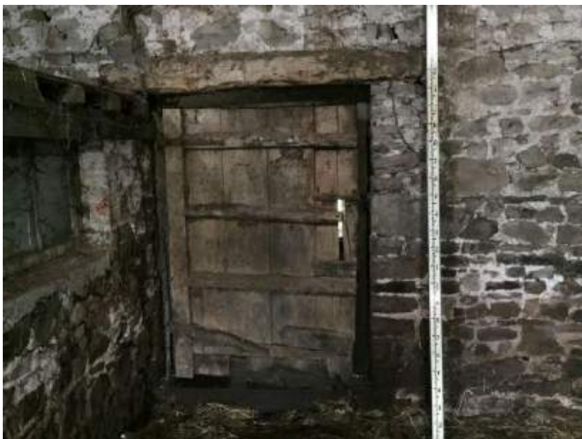
Figure 21 View of doorway and opening to rear shut out shippon with timber lintel over opening.
