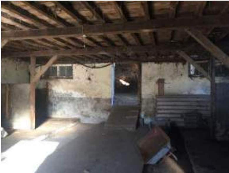
Figure 23 View of doorway and ramped access to lower shippon area, note channels to floor and timber post supports for the timber deck over.
