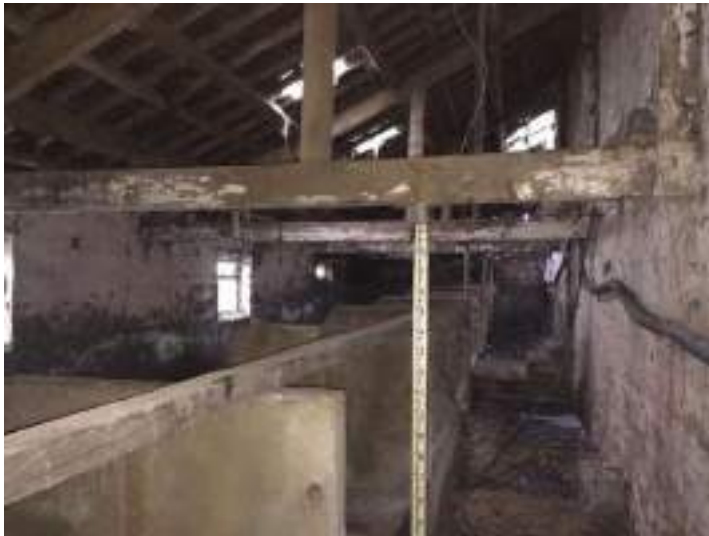
Figure 25 View along rear shippon showing concrete stalls, mono king post trusses and stepped access to main barn.
