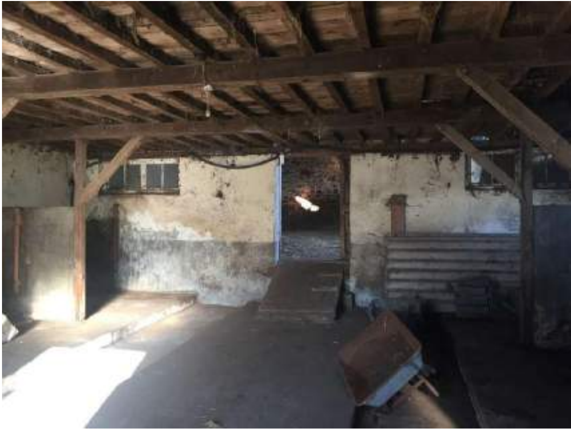
47 View facing internal entrance and ramp into lower shippon, note supports for timber deck above
