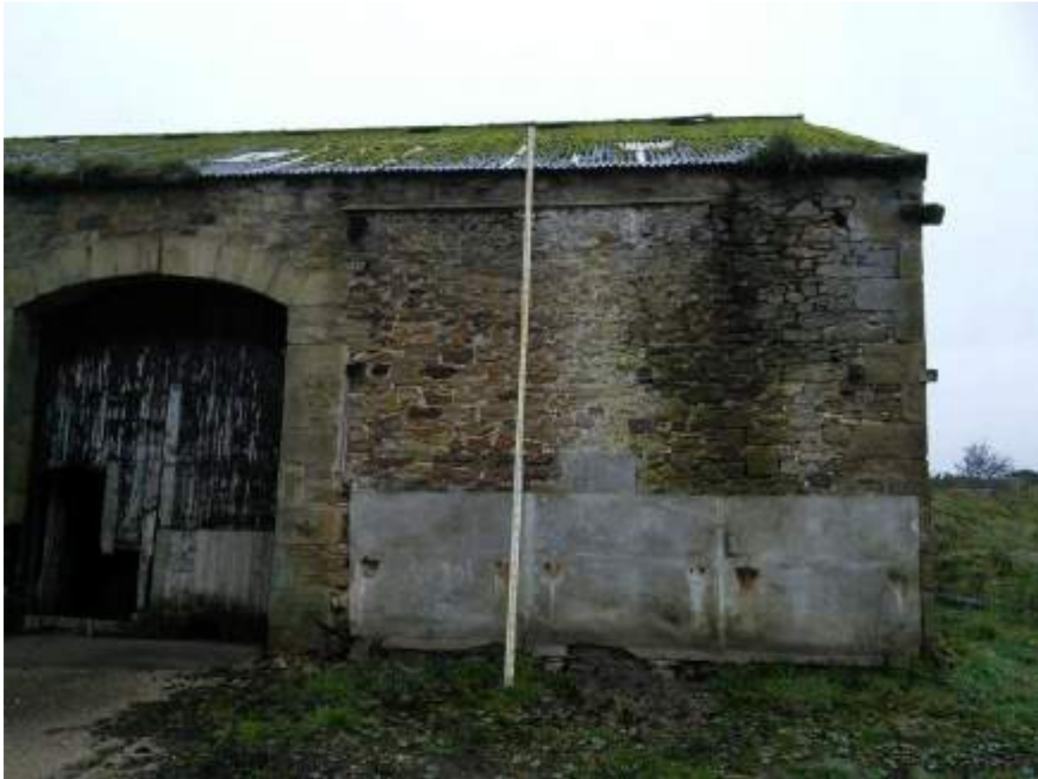
7 Left hand view of front elevation showing render panels applied to stonework. Note timber ends protruding from stonework below eaves level that once supported the timber lean to structure.
