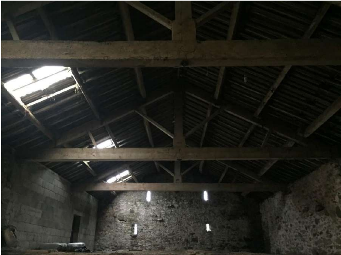
35 View of raised timber deck over shippon, note access was not possible to the level.
