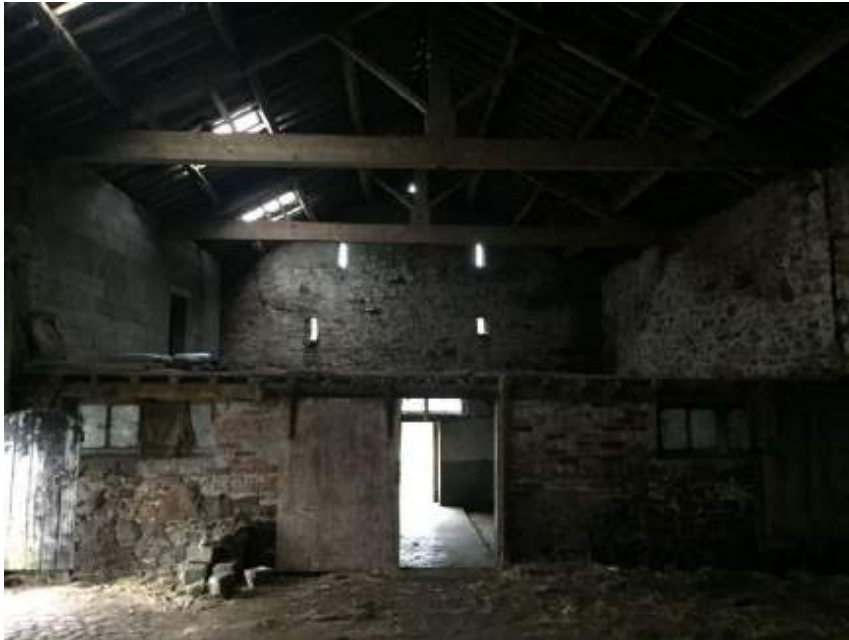
Figure 22 Internal view of the south west elevation showing the timber deck and shippon area below, note matching ventilation slits and owl hole to gable wall. Joggle king post trusses supporting purlin and rafter roof.
