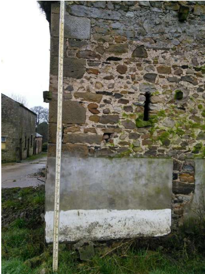
29 left hand corner view showing rendered panel, stone corner quoins and slits within wall.
