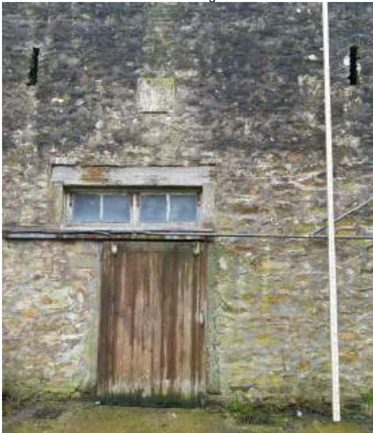
12 Centre doorway, note lack of side stone quoins and head denoting possible later addition.
