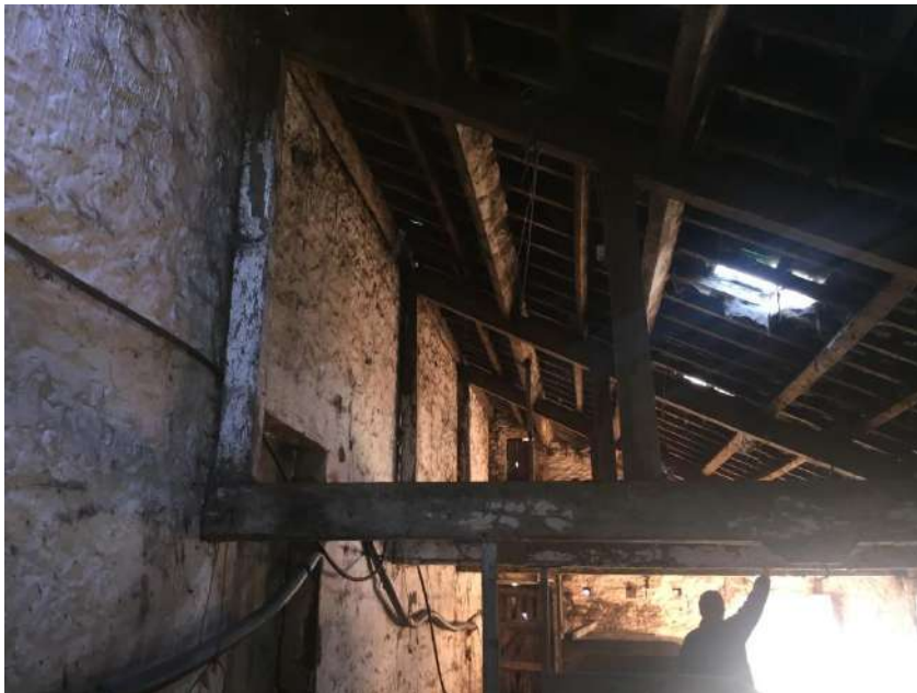
60 Detail of trusses showing metal poles supporting the two central trusses either side of doorway.
