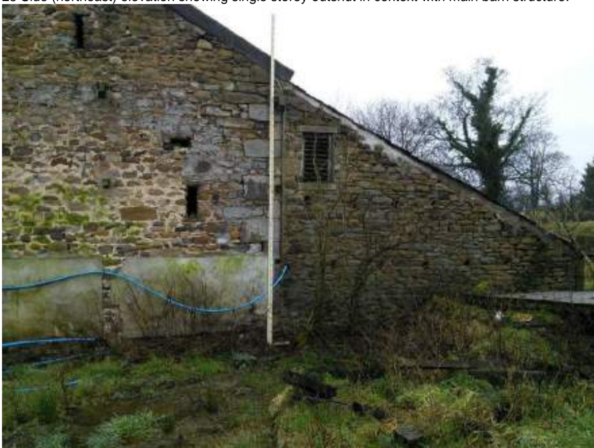
26 View of corner quoins, note ventilation slits and timbers jutting out from wall at high level that formerly supported the roof to the timber lean to structure that was formerly attached to the barn.
