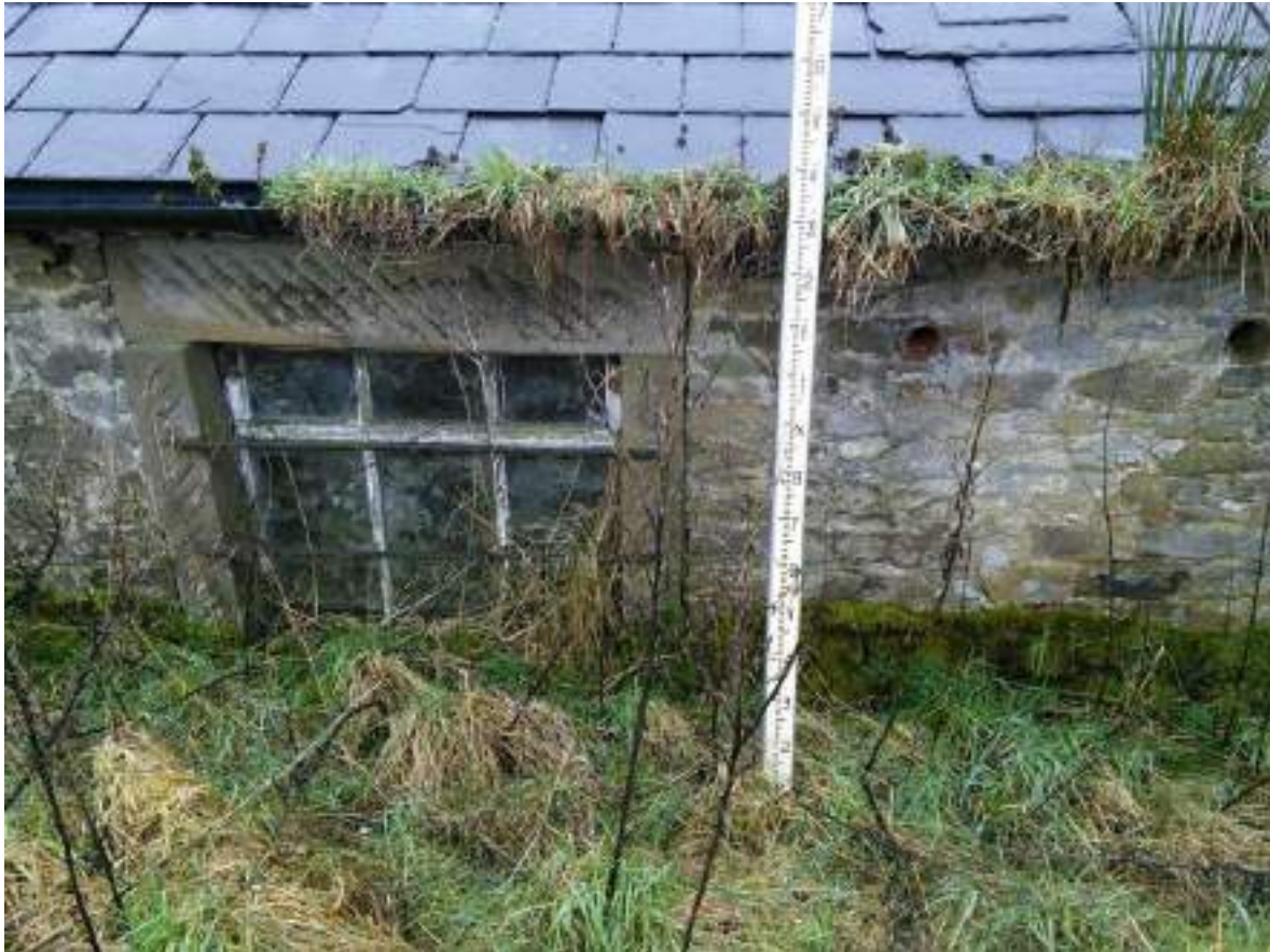
21 Window detail to rear elevation with boasted stone surrounds. Note ventilation holes at eaves level.
