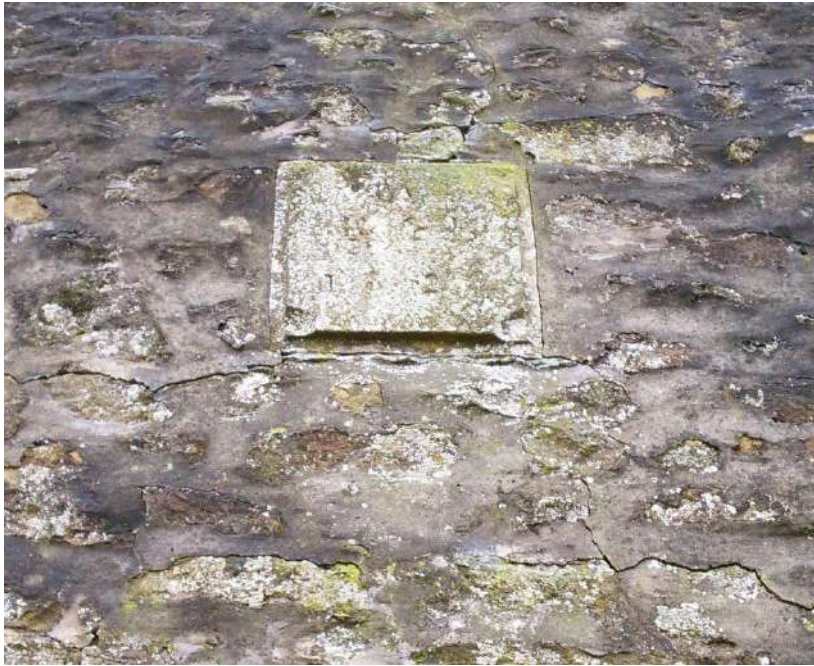
Figure 13 Stone plaque to the south west elevation, visible are the numbers 18 2? Possibly relating to the build date.
