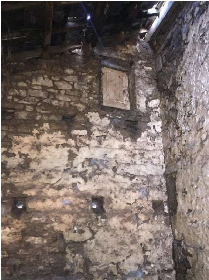
59 Internal view of high level louvered vent showing internal door to block off the ventilation.
