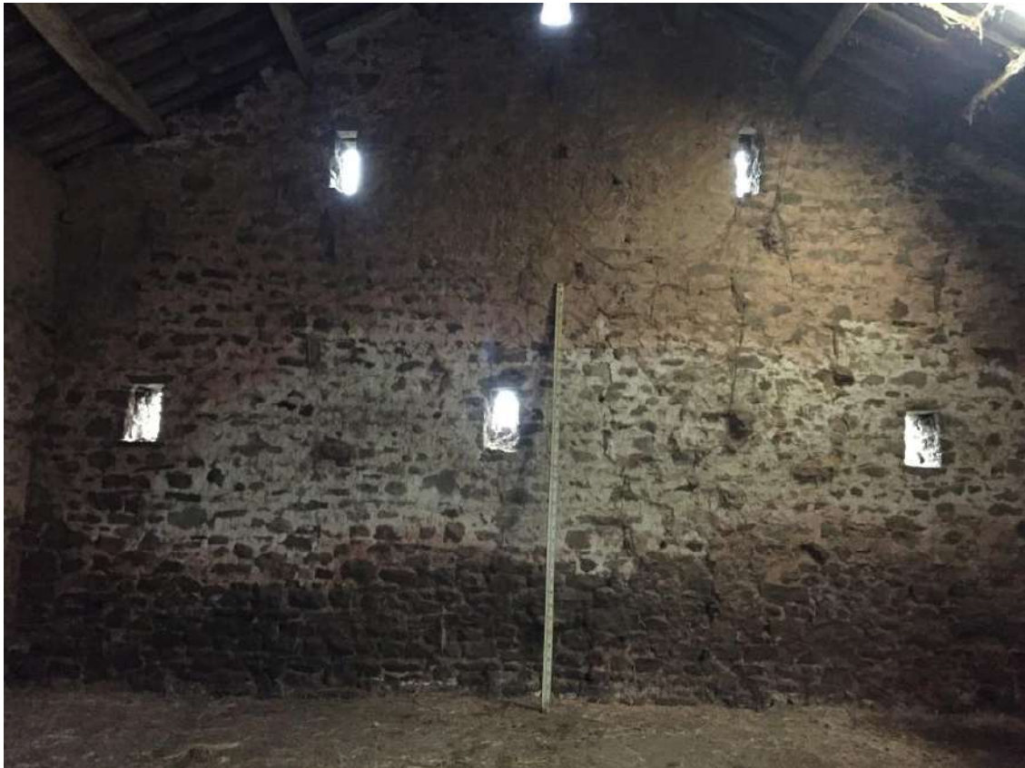
43 View of northeast gable elevation showing ventilation slits and owl hole close to ridge
