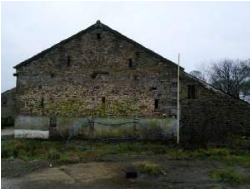
Figure 17 North east elevation of Barn Two showing the rendered panels applied to the gable wall.
