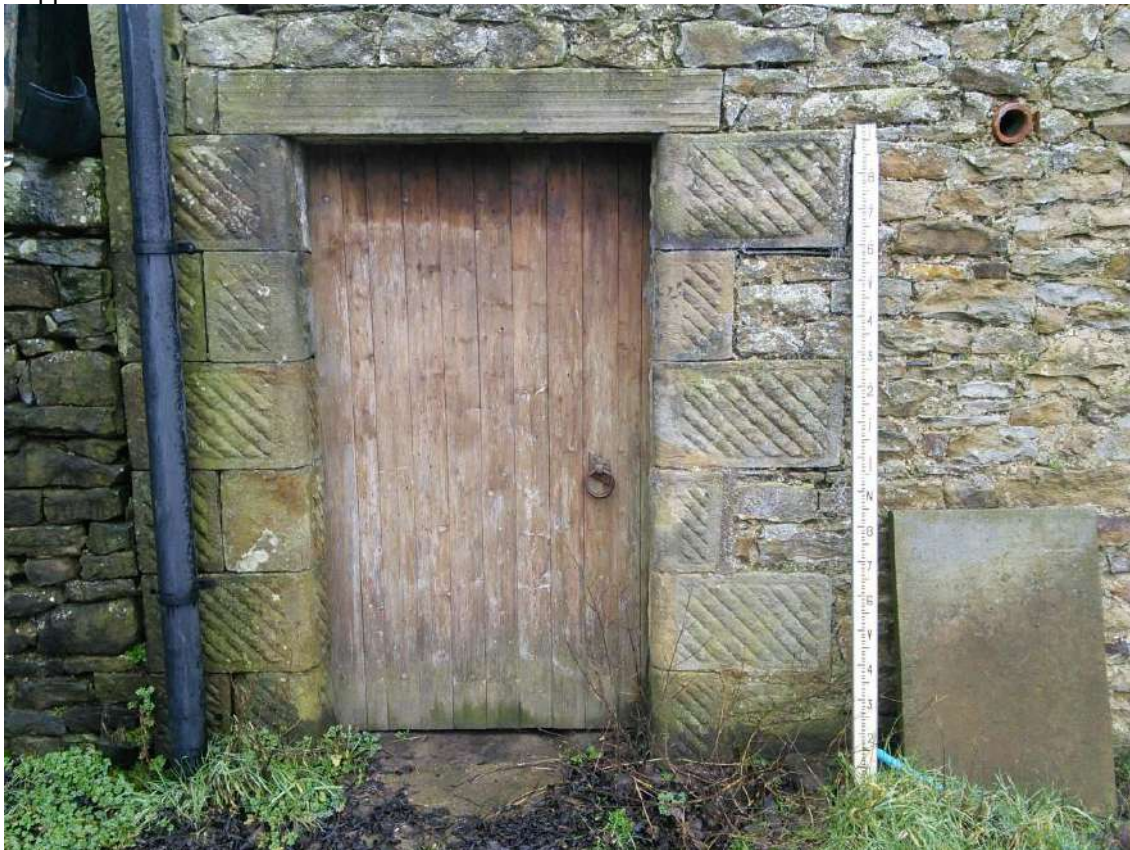
16 View of left hand door providing access to rear shippon, note curved quoins with boasted finish.
