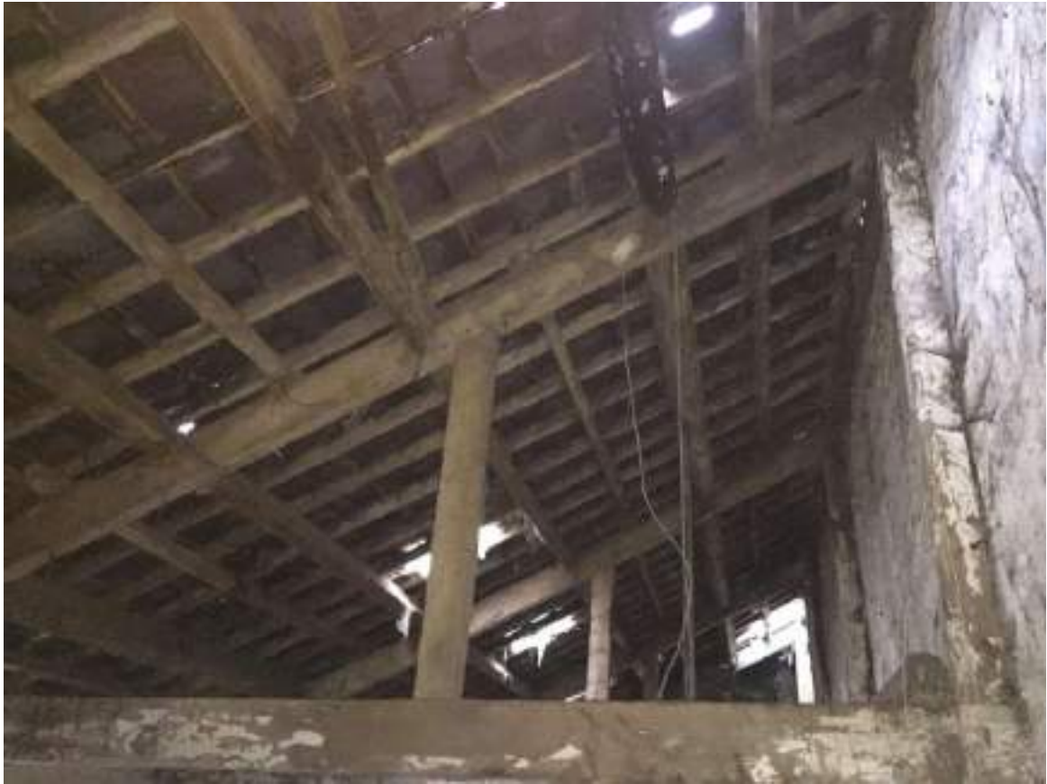
55 Mono pitch king post trusses to outshut with primary and secondary purlins supporting roof rafters.
