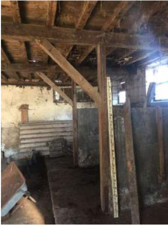
49 View of post and strut supporting beam with joists and boarding over.
