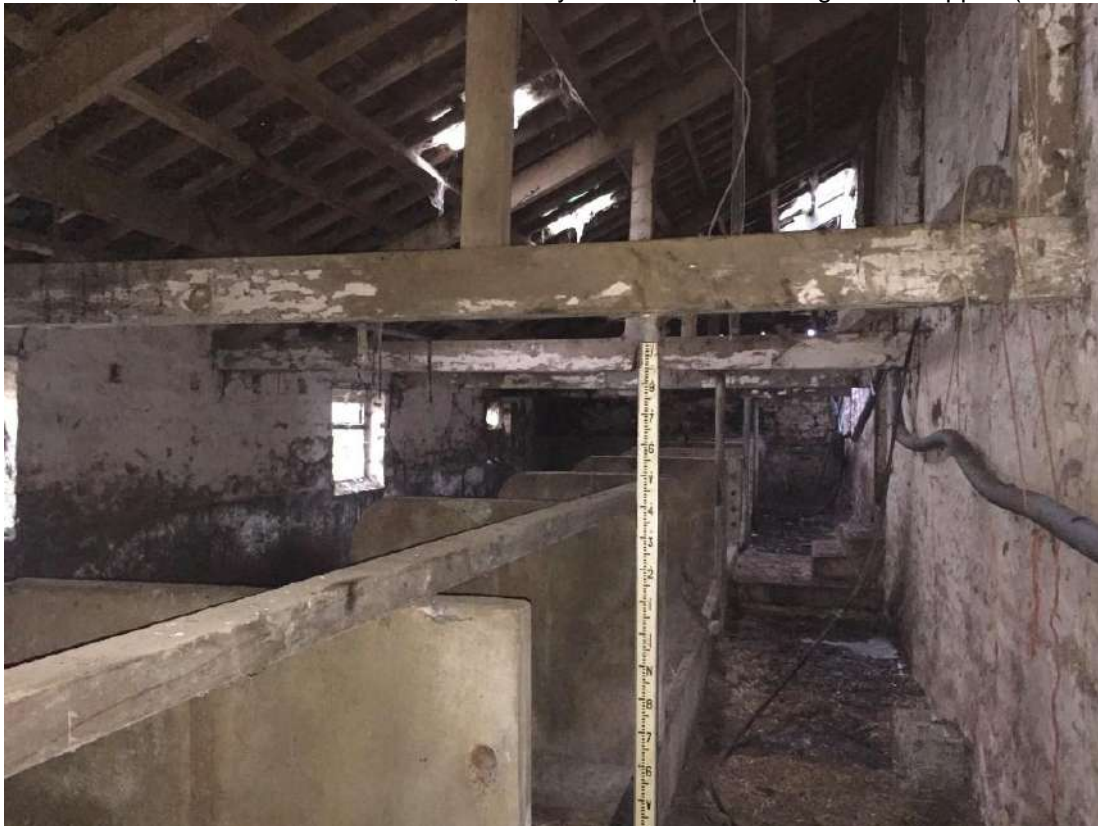
54 View along lower shippon area showing cattle stalls and stepped access from main barn.
