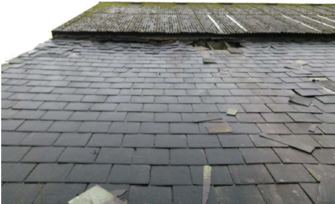
23 Rear view of outshut roof covering showing damage to roof finishes, note slates are a modern addition and not original.
