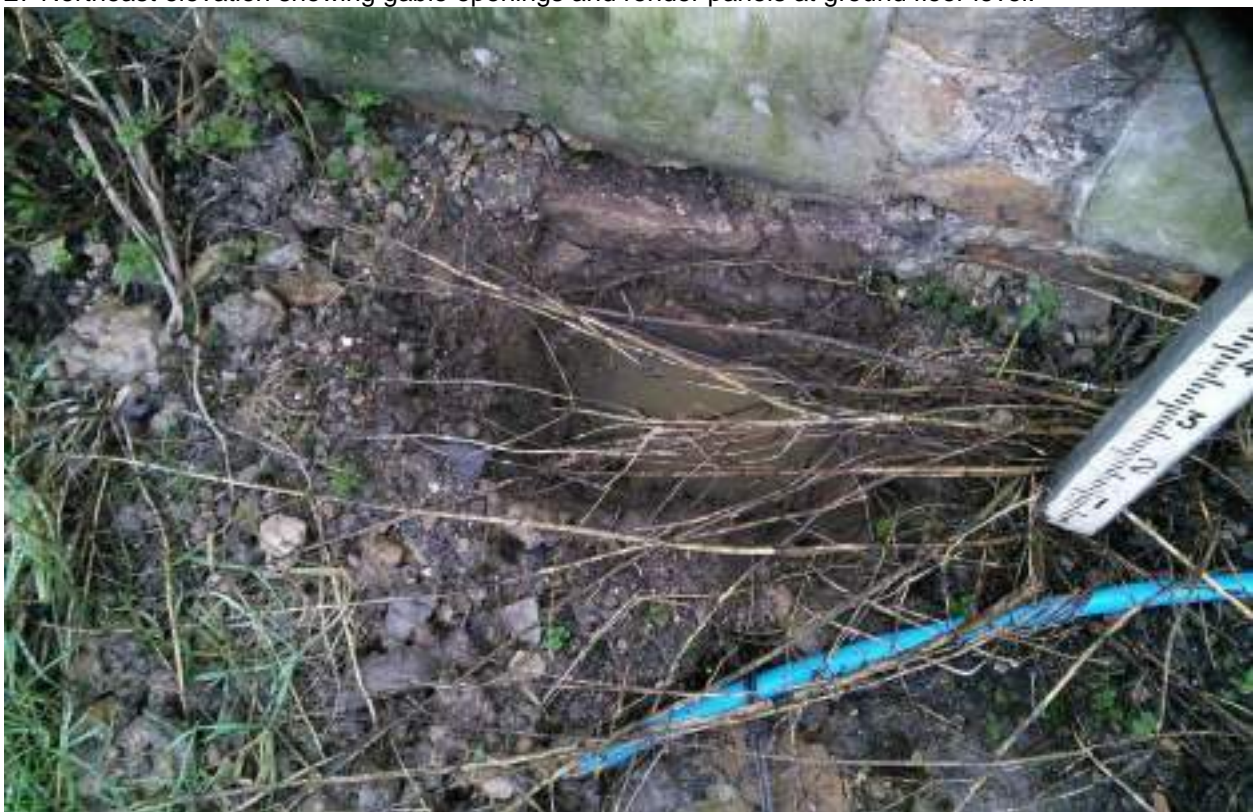
28 View of a trial hole excavated adjacent to wall to ascertain the foundation type and depth.
