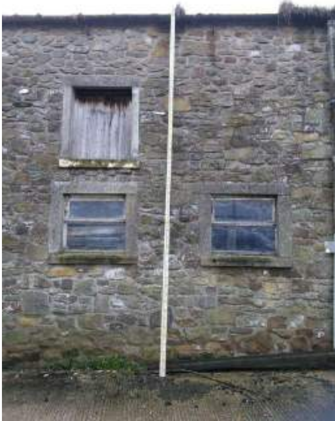
3 Window detail to lower level shippon with hayloft door above, note window surrounds appear to be precast units and may have been a later addition.
