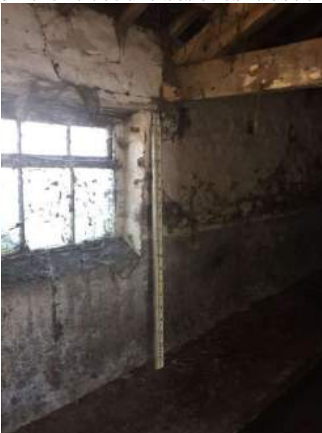
58 North west rear wall showing window with render to cill level, note sloping window cill to window
