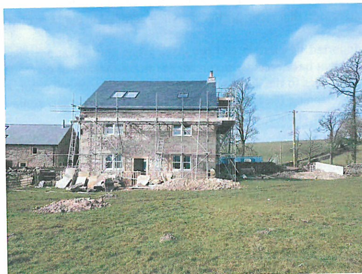
Abbot Barn Farm – looking west and showing the new roof. Note the similarities in the roof of the recently converted barn in the background
