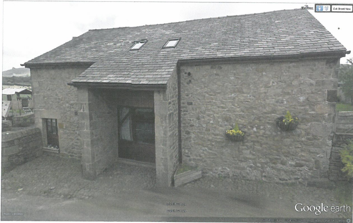
PLATE 7 RANDOM STONE EXISTING WEST ELEVATION DETAILS TO BE COPIED ON THE WEST ELVATION MATCHING IN NEW SUN LOUNGE EXTENSION.
