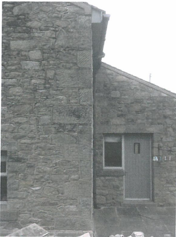
PLATE 4 1 WEST GABLE STONE QUOINS VARY IN SIZE 400MM X 600MM X 200MM VARY IN SIZE TO BE COPIED IN NEW EXTENSION SURFACE OF STONE QUOINS TO HAVE A TOOLED FINISH TO MATCH EXISTING
