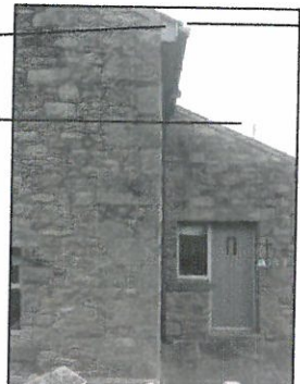
PLATE 4 Existing sandstone stone work detail walls random with stone course dressed stone quoin and eaves details
