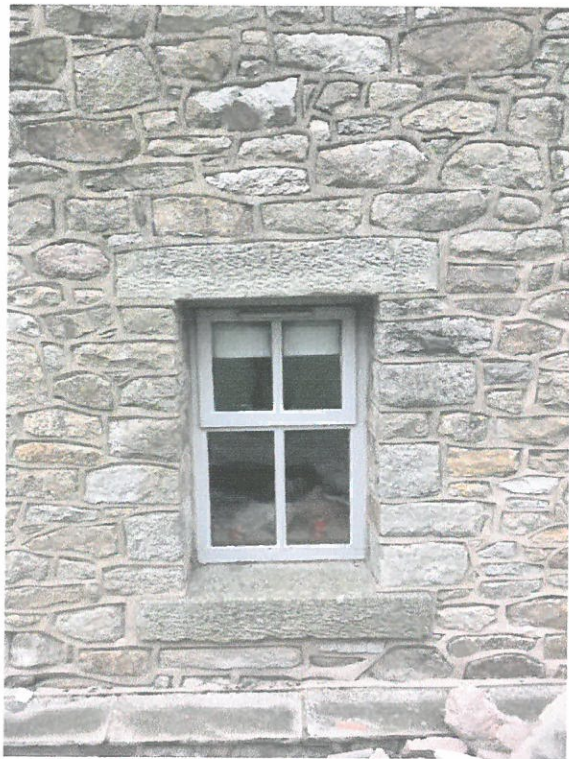
PLATE 6 RANDOM STONE & WINDOW DETAIL ON EXISTING SOUTH ELEVATION DETAILS OF REVEALS TO BE COPIED IN NEW SUN LOUNGE EXTENSION. NEW TIMBER WINDOW SASH FRAMES TO MATCH EXISTING PAINTED TO MATCH EXISTING. STONE HEADS 200 MM TO 240MM ON FACE DEPTH EQUAL TO THICKNESS OF STONE 150MM
