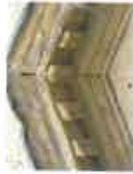
P1220436 - Chipped arris
