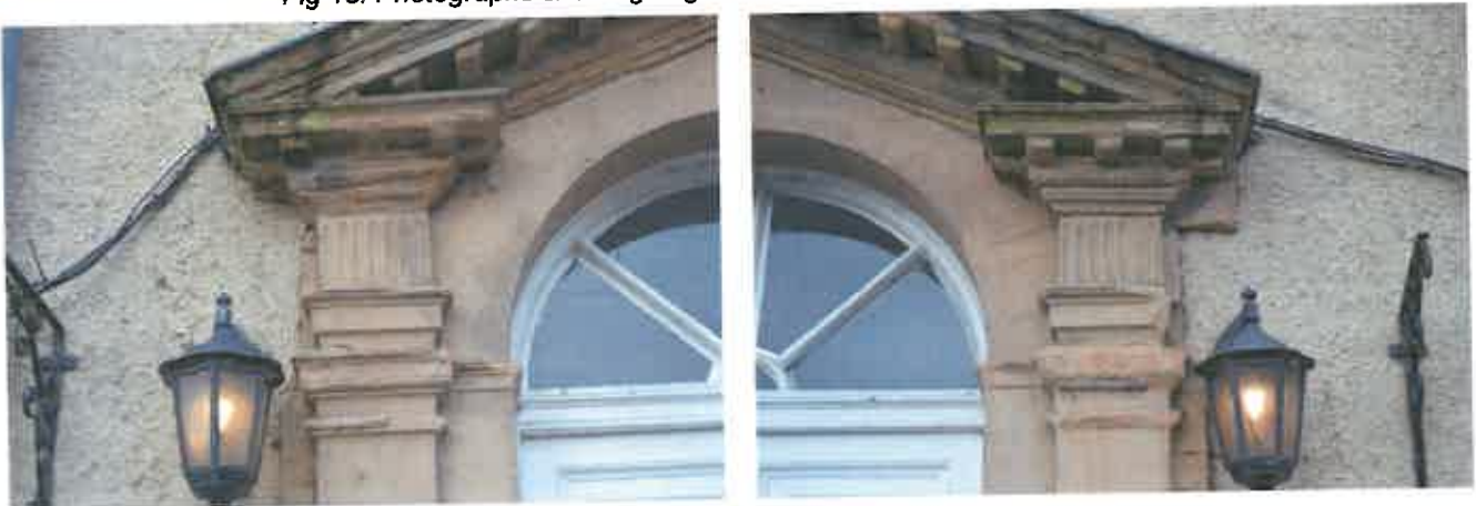
Fig 16: Photographs showing degradation to the pilaster capitals.
