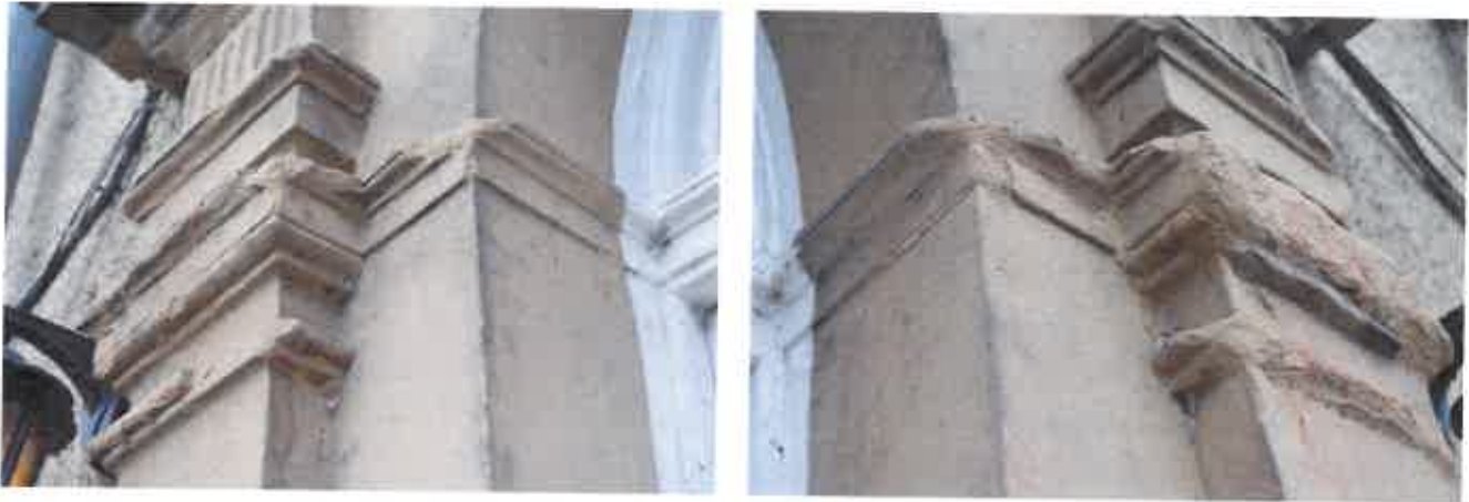
Fig 18: Photographs showing degraded arisses.
