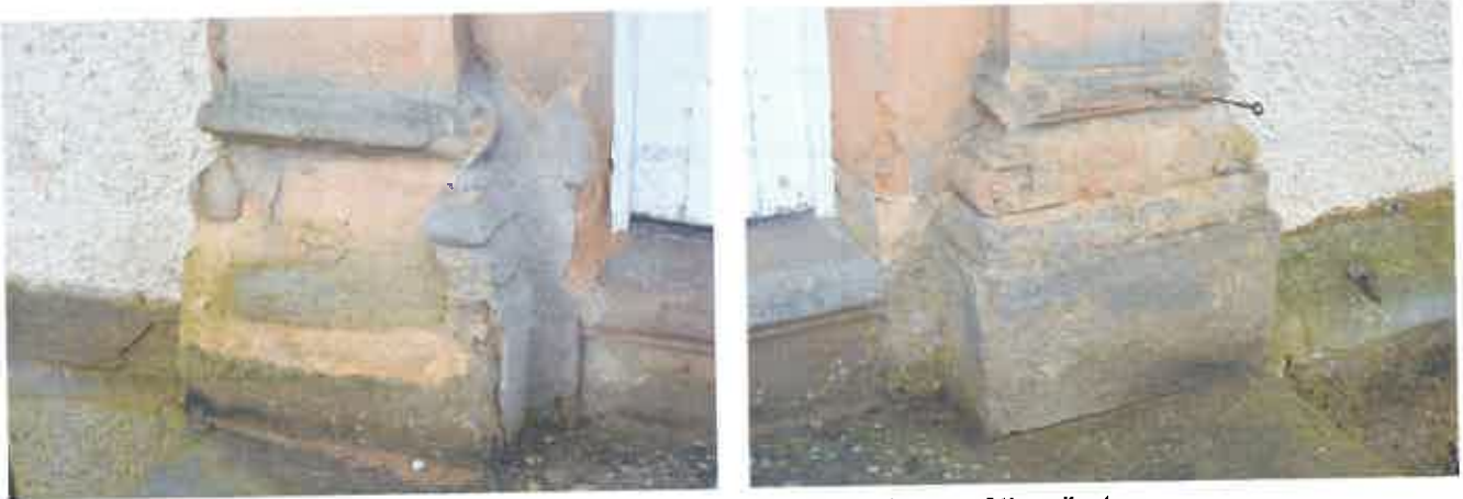
Fig 15: Photographs showing degradation to the bases of the pilasters.
