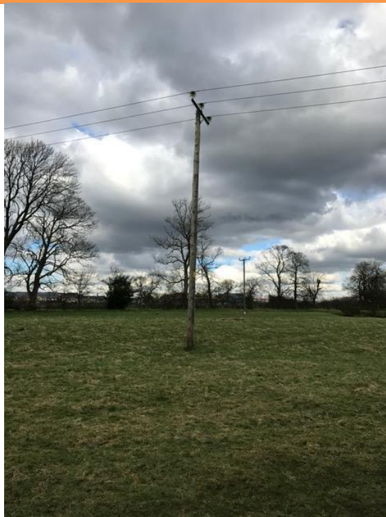
PLATE 2 – OVERHEAD ELECTRICITY CABLES IN WEST SECTOR
