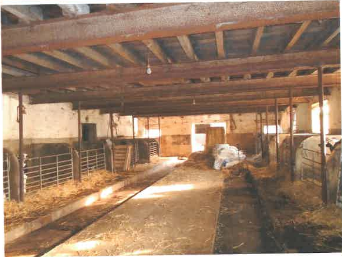
Photographs (24 - 26) – Illustrating the floors visible / condition of the floors within the barns.
