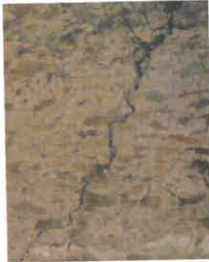
Photograph (12) – Showing the crack within the Storage Area.
