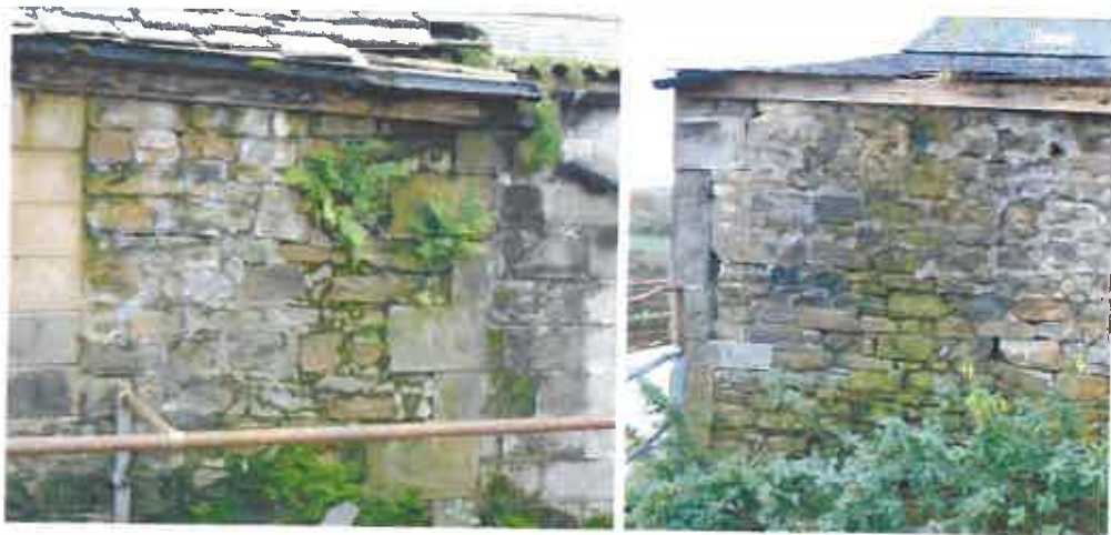
Photographs (14 and 15) – Showing the external corners to the lean-to which need re-building.
