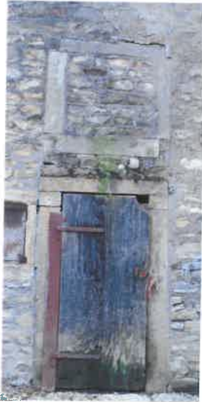
Photograph (13) – Showing the Store wall which needs re-building.
