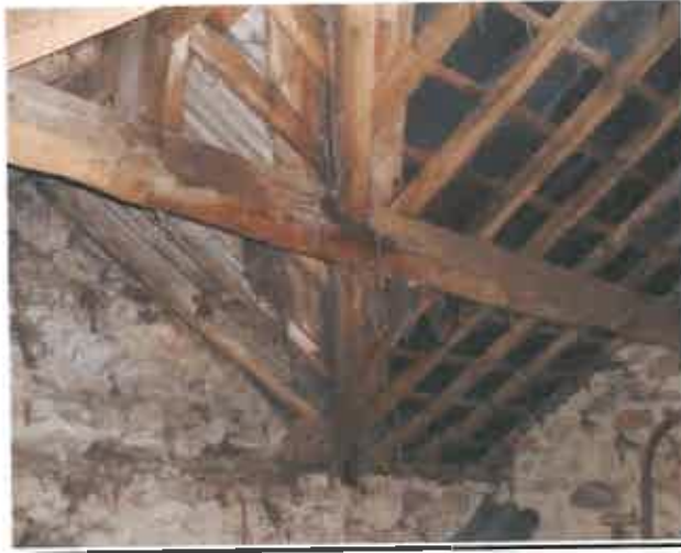
Photograph (3) – Poor condition of roof junction to the South West and North East barn.
