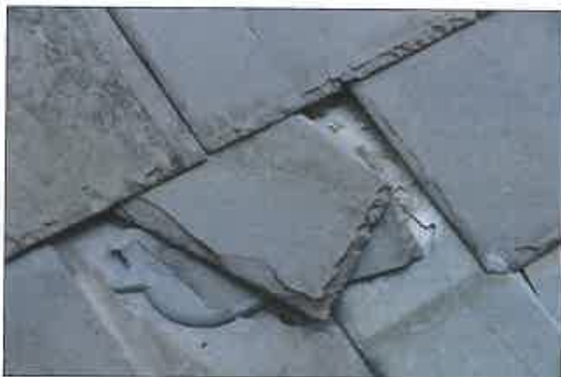
Slipped and broken slates – potential access point for bats
