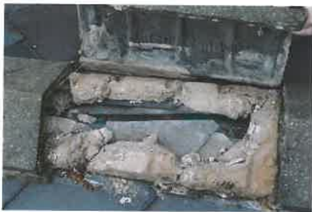
Lifted ridge tile showing unmortared section beneath – potential bat roosting feature
