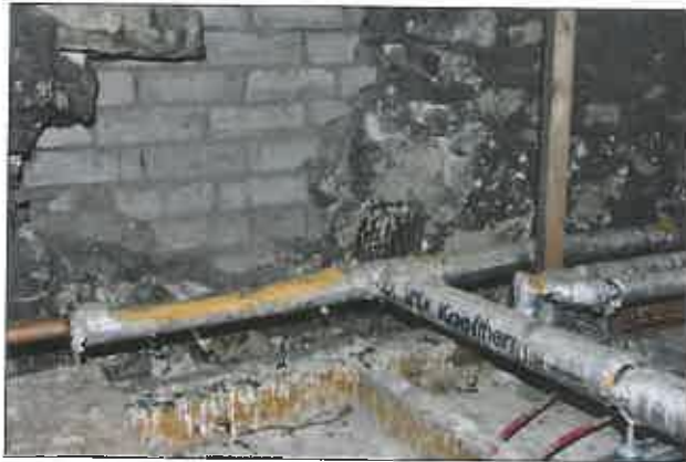
Clear signs of previous pigeon infestation in roof void
