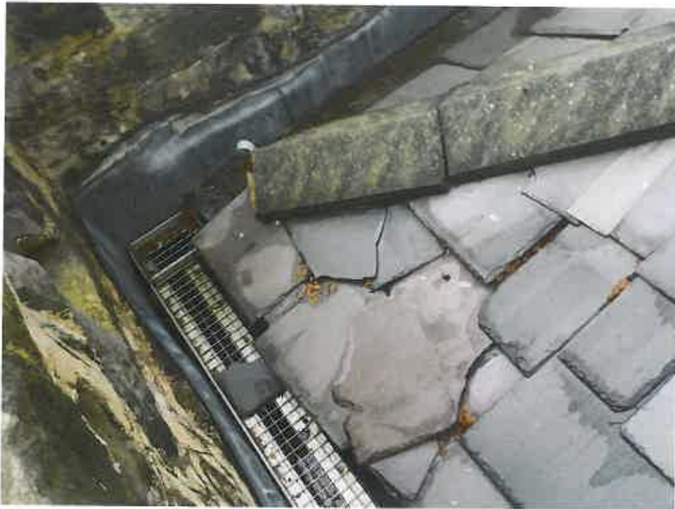
Figure 2 – Shows damaged slates around the perimeter of the pitched roof in the area of the parapet gutter. It is also clear that different slate types have been used.
