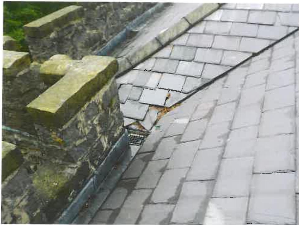
Figure 3 – further evidence of broken slates and different slate types
