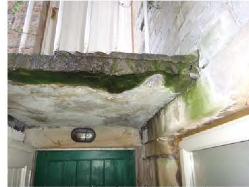
View to underside of existing steps stone landing, showing overlap above basement room window.
