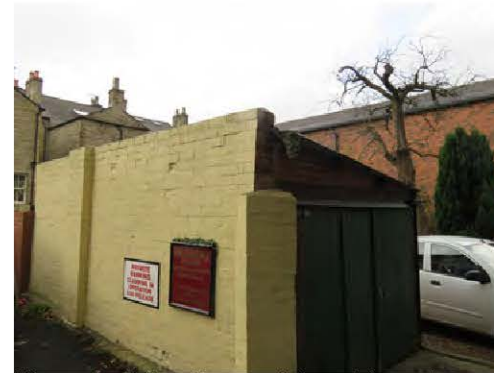
View of existing Garage / shared boundary wall with The Old Post House Hotel, from rear alley.
