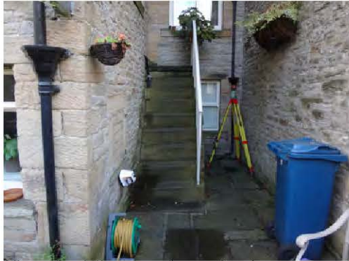
View of existing rear steps, showing uneven stonework treads.
