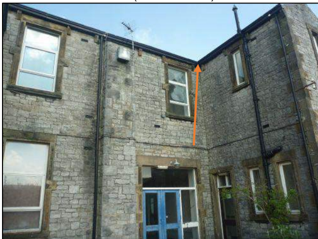
Photo 53: One common pipistrelle emerged from roof edge in the northern corner of the alcove at the southern elevation of Building 3 on 15 th June 2016 11 . It is suspected that one brown long-eared bat was also detected emerging from this location (Roost 2016-C)
