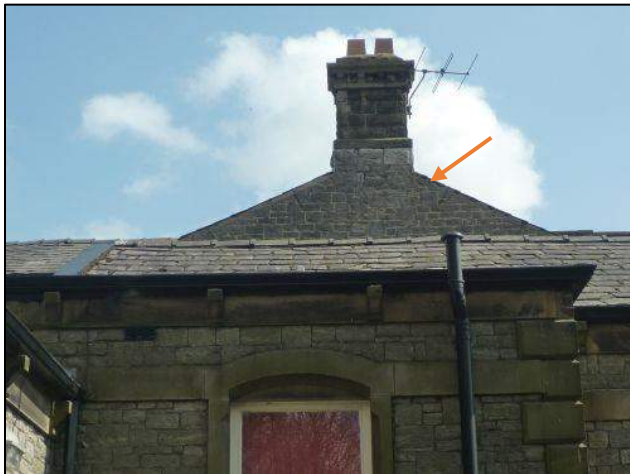
Photo 48: 20 to 30 droppings detected at western gable interior wall of Building 1 in 2008 (Roost 2008-A)
