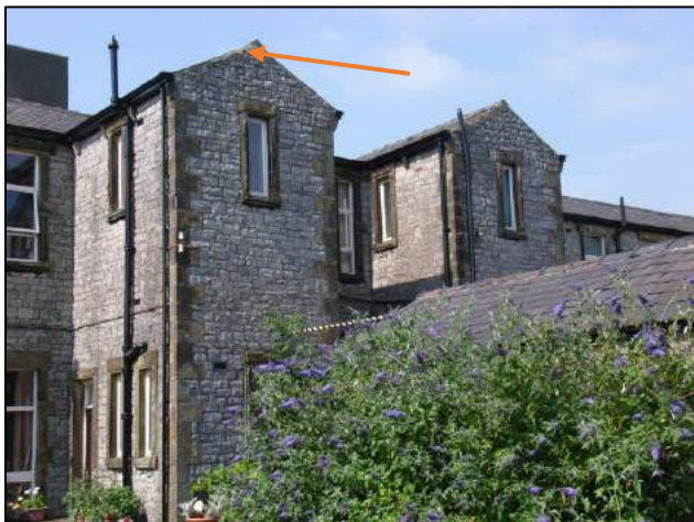
Photo 50: One common pipistrelle emerged from beneath ridge tile at 21:30 on 22 nd July 2008 (Roost 2008-C)
