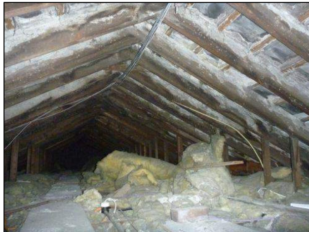
Photo 20: Building 1, roof void above single-storey section of building at eastern end of the building (1d)
