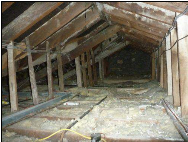
Photo 15: Building 1, northern section of roof void above two-storey section of building (1a)
