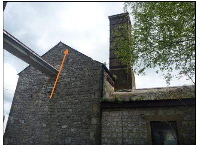
Photo 49: 15 to 20 bat droppings, indicative of pipistrelle bats, present on the upper floor and walls beneath gap in the ceiling below the roof void, at the western elevation of Building 7 (Roost 2008-B)
