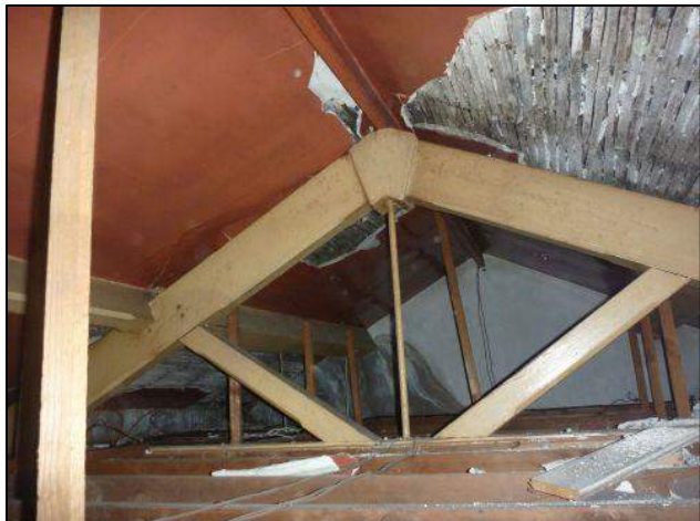
Photo 19: Building 1, roof void above kitchen area, at single storey section at the southern end of the building (1c)
