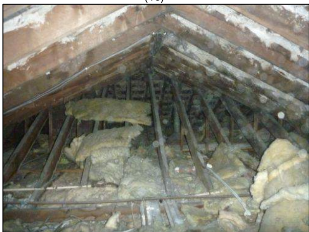
Photo 21: Building 1, roof void at northern end of the single-storey section of the building, at the building's eastern end (1d)
