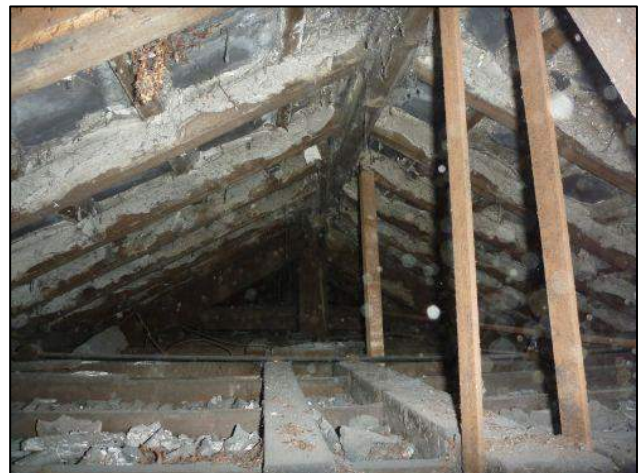
Photo 18: Building 1, roof void above single storey section at south-western corner, shorter section of void (1b)
