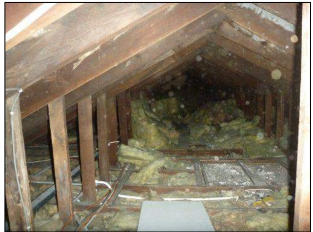
Photo 16: Building 1, southern section of roof void above two-storey section of building (1a)
