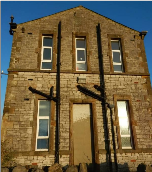
Photograph 8: Gable end return on former Infirmary demonstrating blocked door opening and tripartite windows.
